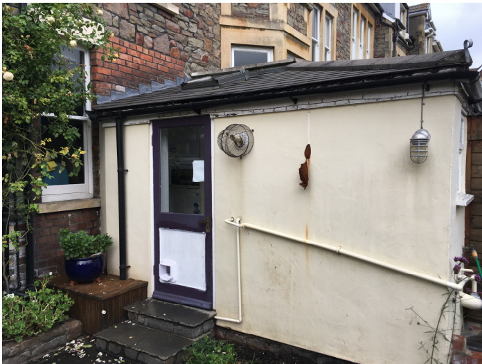
2. Side Elevation view of existing extension towards boundary with no.53 Manor Park
