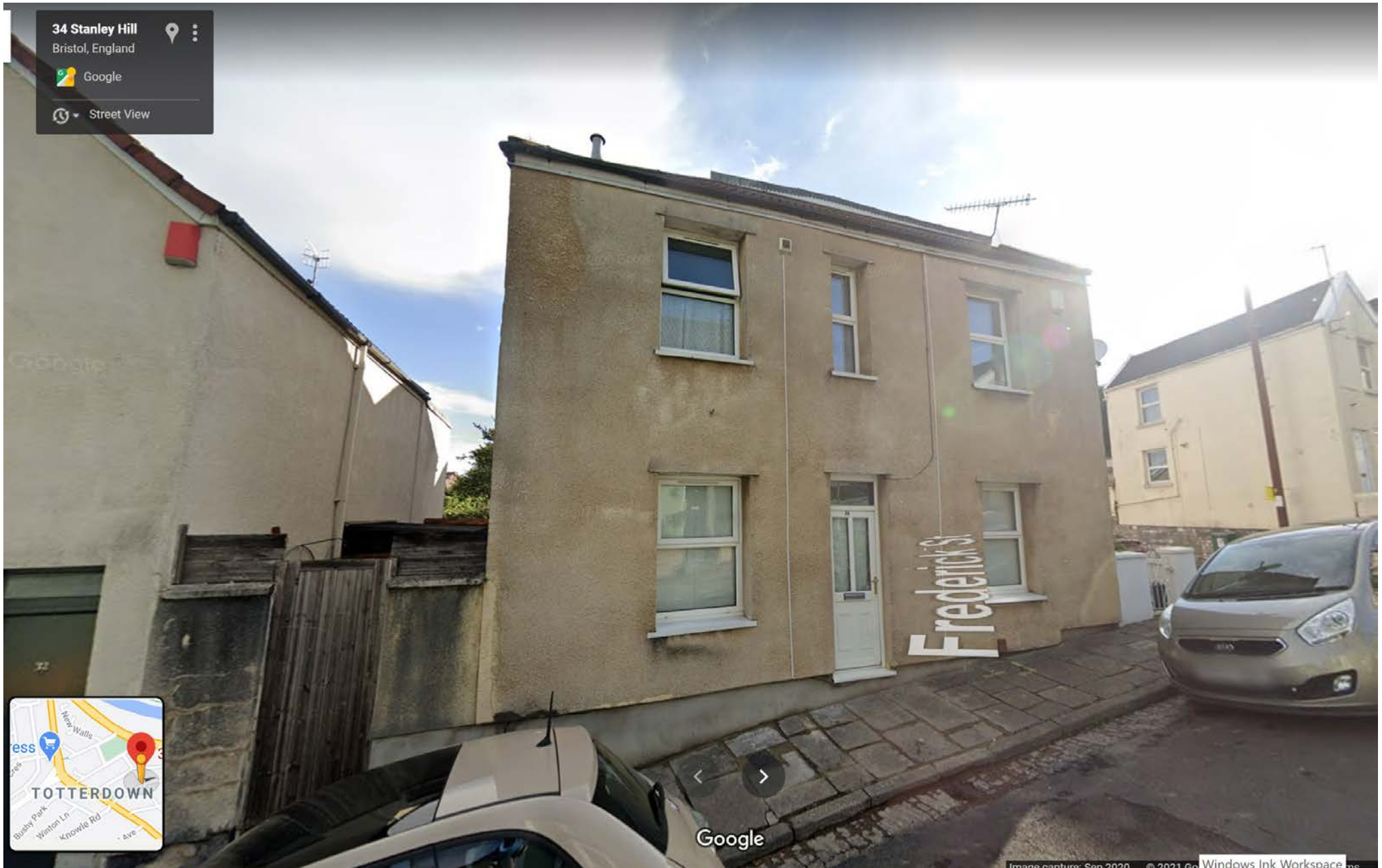
View of 34 Stainly Hill, Front elevation. An external insulated render had been added in the past.
