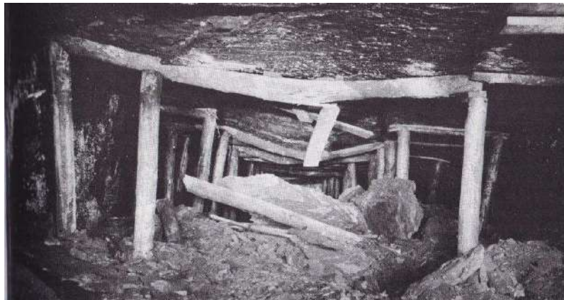
Typical settlement in a timber supported roadway
