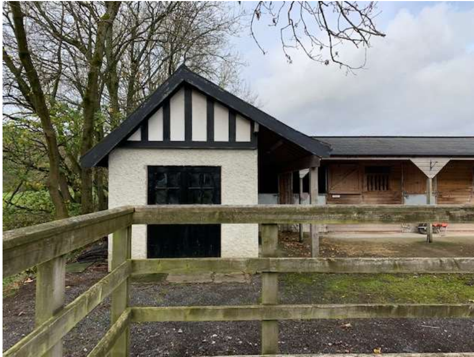
Existing masonry building attached to timber stables to be retained and insulated to form a drying room
