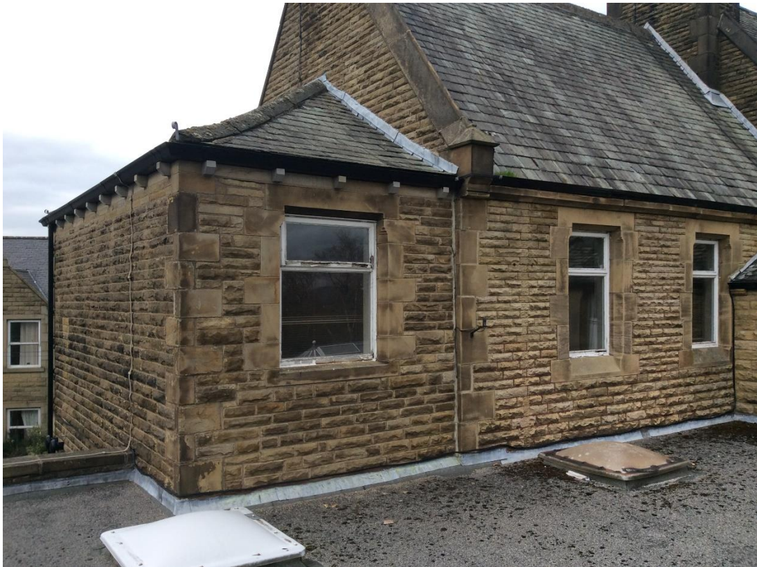
Example of rotten windows
