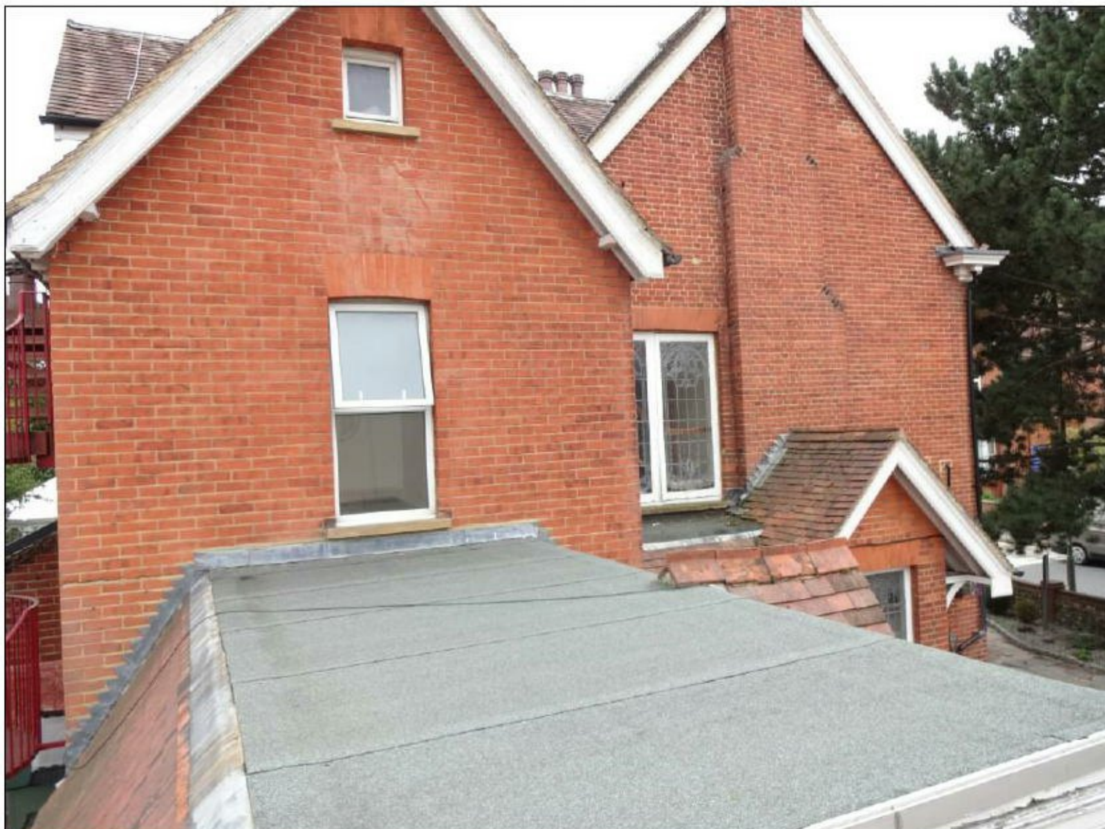
Figure 8. Example of flat roof, Epsom Lodge Care Home, Epsom. 09.09.2020
