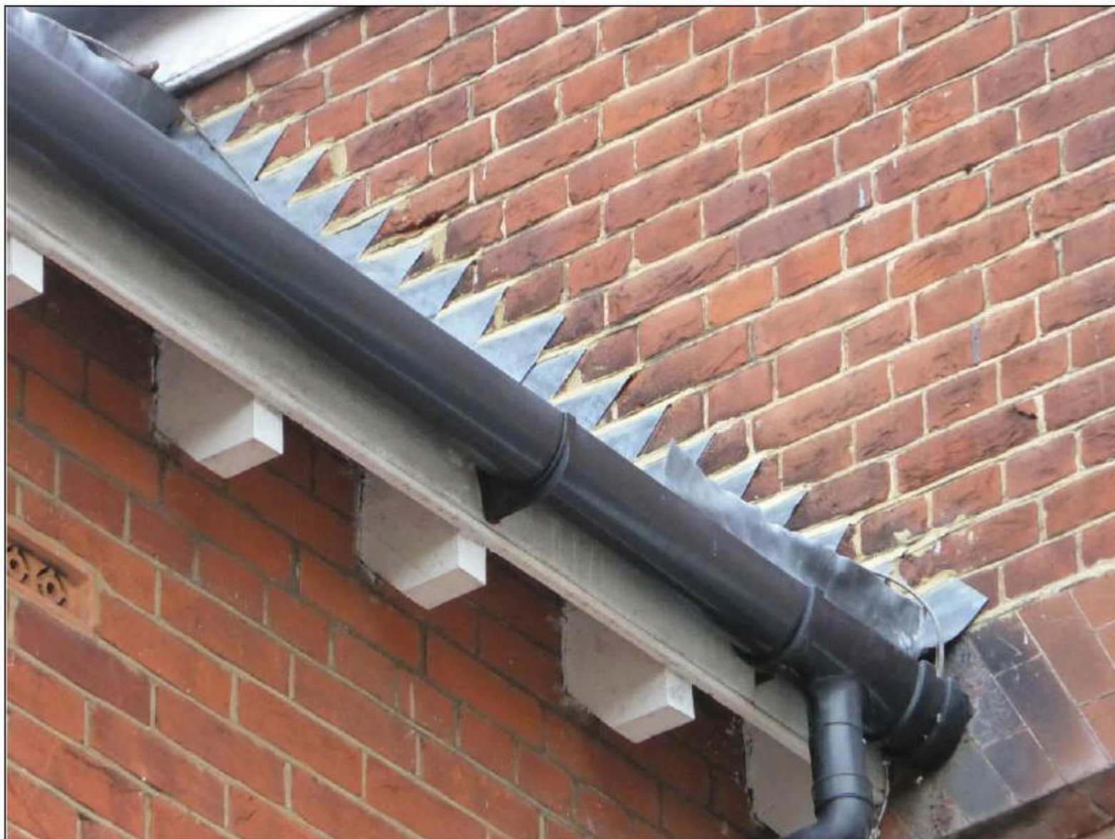
Figure 6. Example of lead flashing between the main building and single storey section. Epsom Lodge Care Home, Epsom. 09.09.2020
