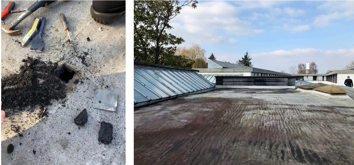
Fig 4 - Photographs of roofs and investigation hole prior to Block D re-roofing works
