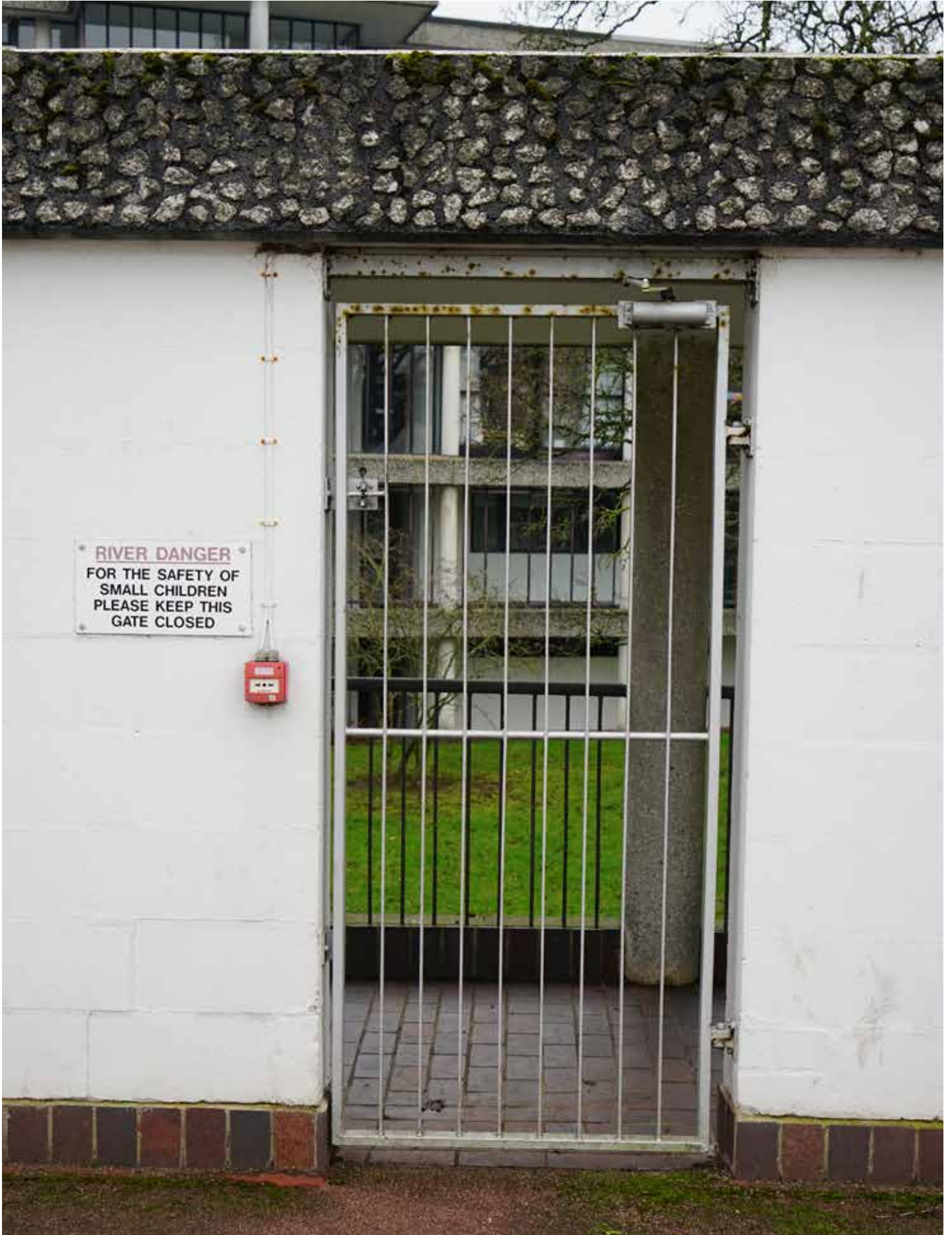
Full height gate with vertical rails and single horizontal rail at mid height at second floor steel. Painted silver, likely to have been black originally.
