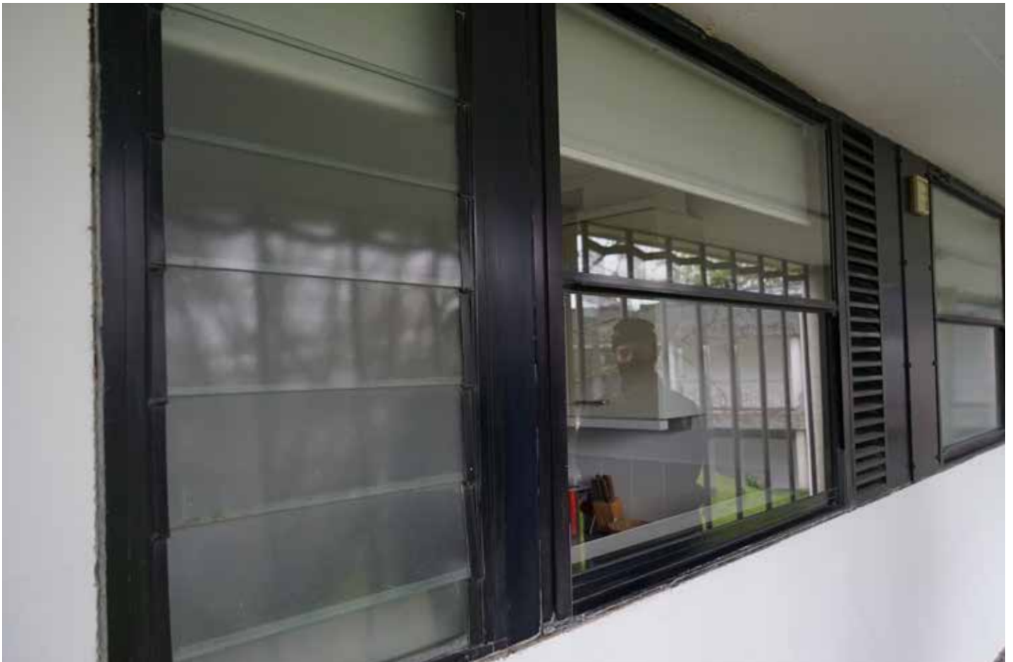
Half height vertical sliders with Aluminium fixed louvres and glass on glass opening louvres to kitchen and bathroom spaces on first floor.
