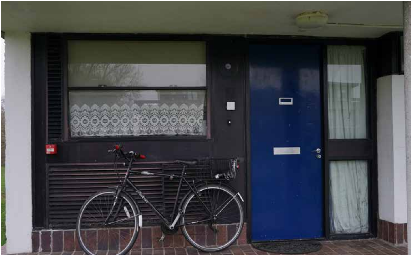
Half height fixed panes either side of central aluminium horizontal brace alongside front doors
