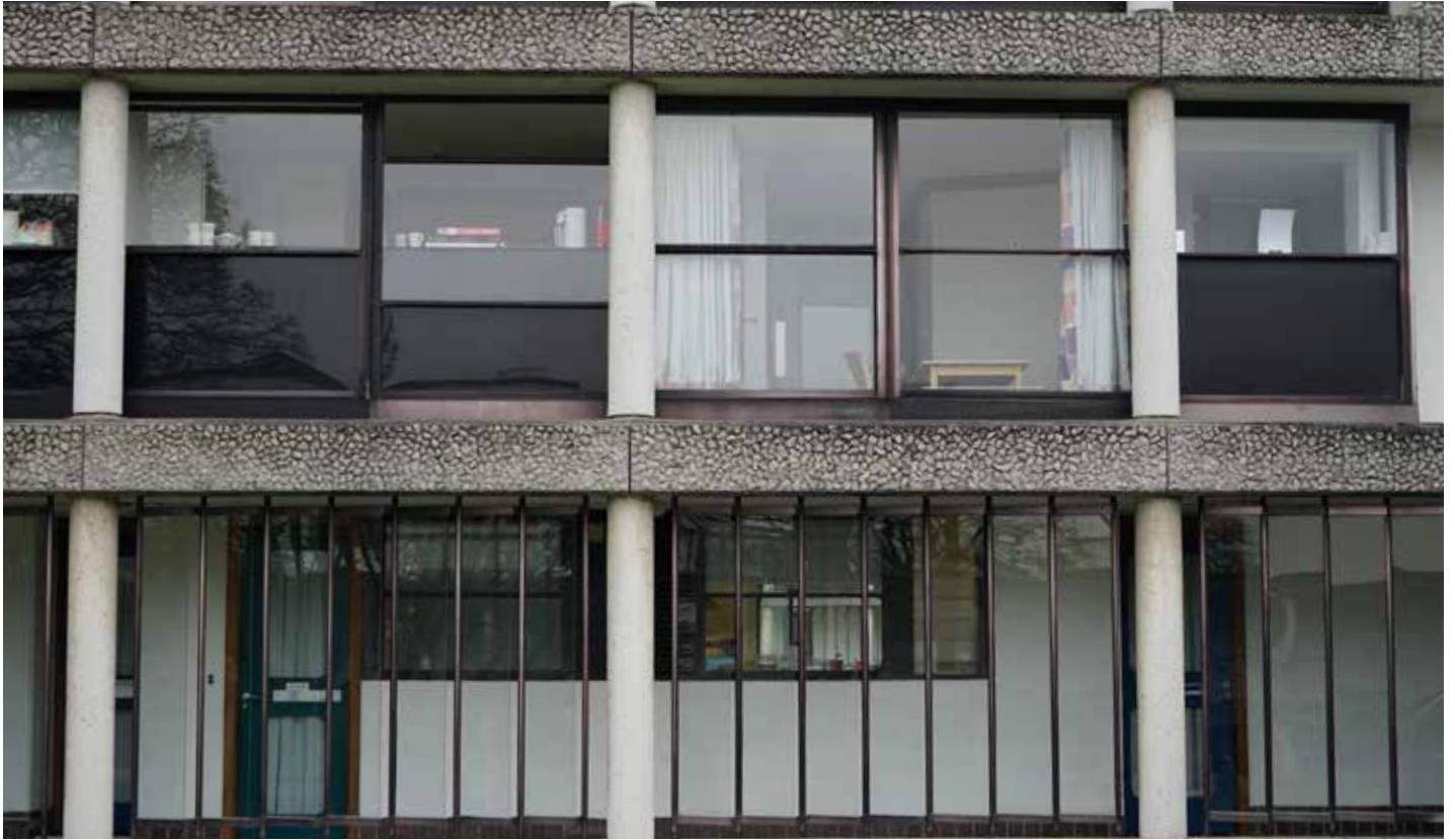
Full height fixed panels in louvred aluminium frames, separating the corridor from the courtyard at first floor level.
