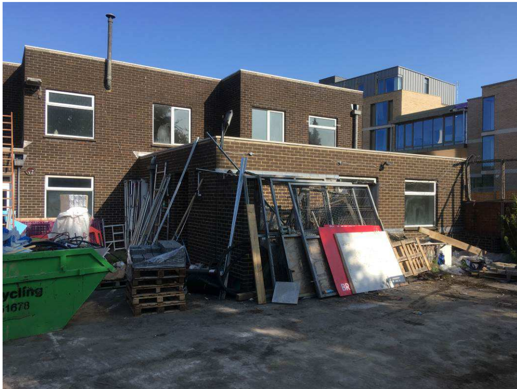
Plate 4 – View of rear of club building looking north-west from club car park.
