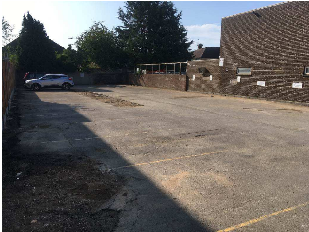
Plate 6 – View of car park for Nos 17/17a Between Towns Road looking south-east. Club building is on right hand side. Scarring on surface of car park evident .
