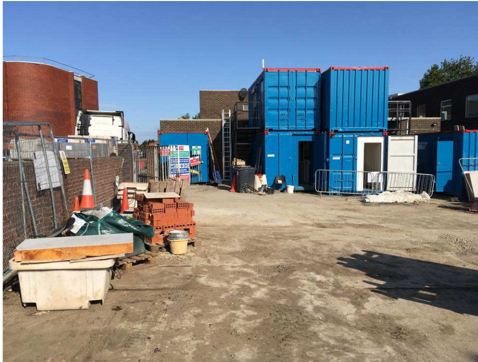
Plate 1 – View from Cowley Conservative Club car park looking west towards rear of club building. Cabins and stores are in use as site compound for development to north of site boundary.
