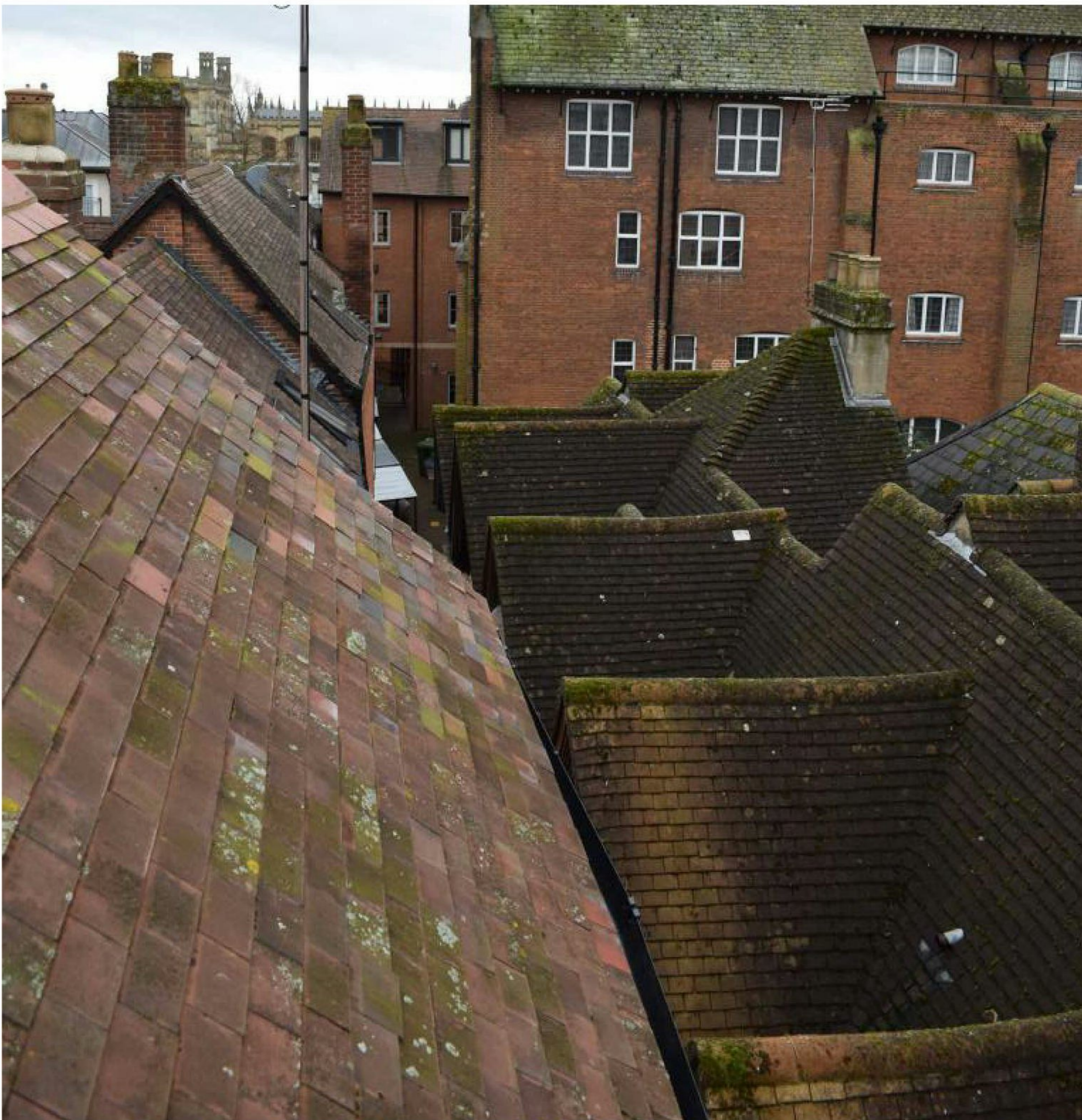
View looking along the roof from the north with the lower area of roof it is proposed to raise. Roof of Kemp Hall to the east (RHS)
