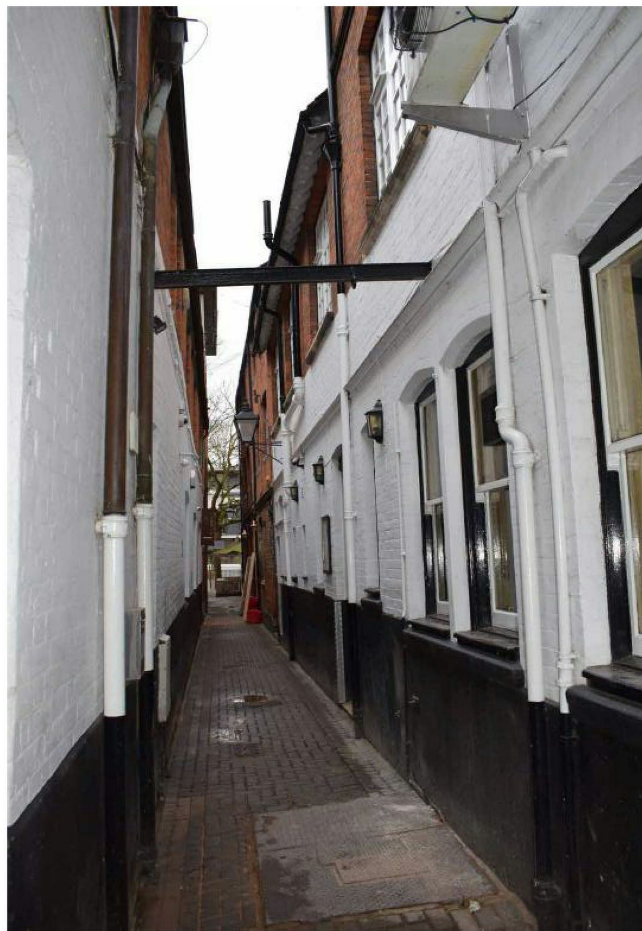
View looking south towards Blue Boar Street showing The Wheatsheaf (RHS) The area of roof proposed to be raised is the portion of projecting eaves
