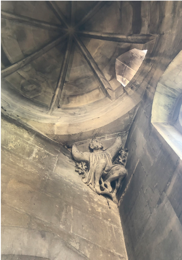
Plate 49 Detail of the stone domed roof and carved figure in the roof of the stairwell, room ST1, 2019 (Donald Insall Associates)
