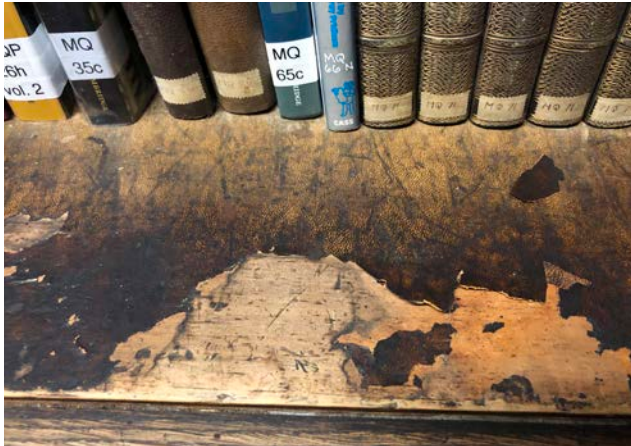
Plate 53 Detail of the damaged original leather lined bookcases, room F1, 2019 (Donald Insall Associates)
