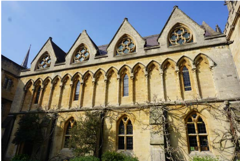
Plate 26 Front (south) elevation of the main Library facing onto the Fellows' Garden, 2019 (Donald Insall Associates)
