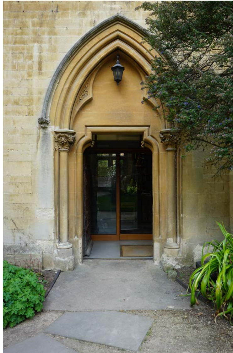
Plate 27 The main (south) entrance into the Library showing the detracting modern glazed lobby behind, 2019 (Donald Insall Associates)
