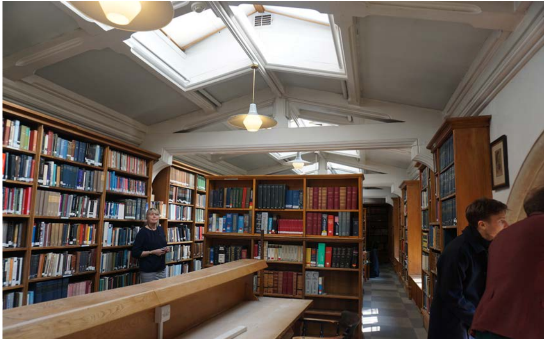
Plate 46 The modern bookshelves and original timber ceiling in the mezzanine. The rooflights are modern additions, as are the painted roof panels, room M1, 2019 (Donald Insall Associates)
