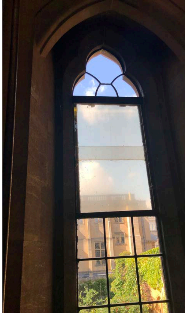
Plate 55 The modern Perspex replacing the original leaded lights in the central north-facing window, room F1, 2019 (Donald Insall Associates)
