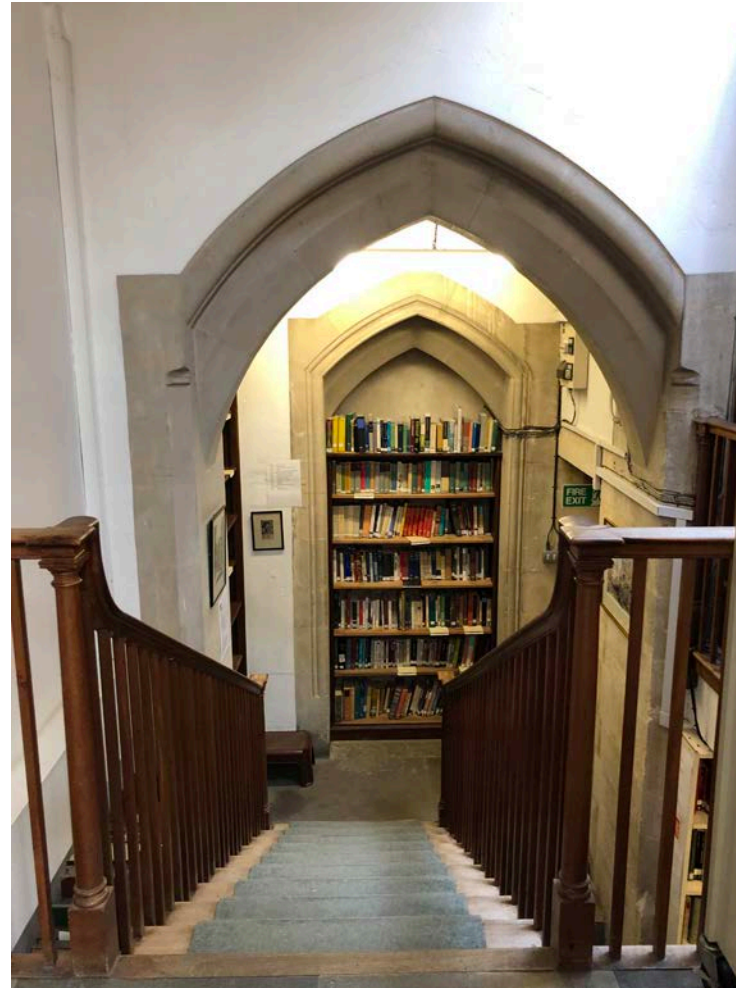
Plate 45 The blocked doorway in room G3 and the modern staircase to the mezzanine, ST2, 2019 (Donald Insall Associates)
