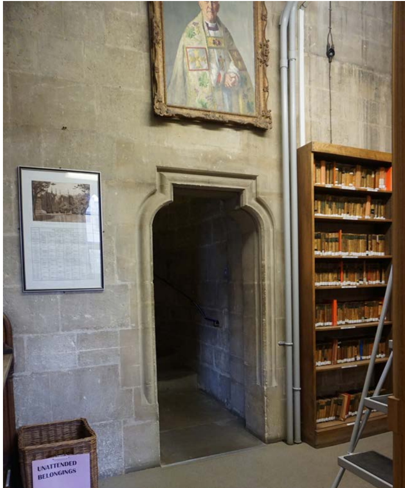
Plate 44 The doorway to ST1, which has lost its original door, 2019 (Donald Insall Associates)
