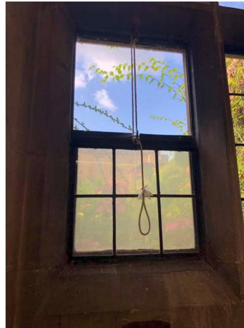
Plate 42 The lost sections of glazing in the ground floor windows, most probably a result of the louvers that were added in 1947, room G1, 2019 (Donald Insall Associates)
