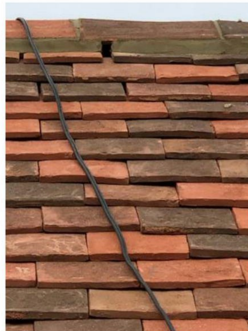
Figure 11. Example of a bat ridge tile set below the ridge, giving access below.
