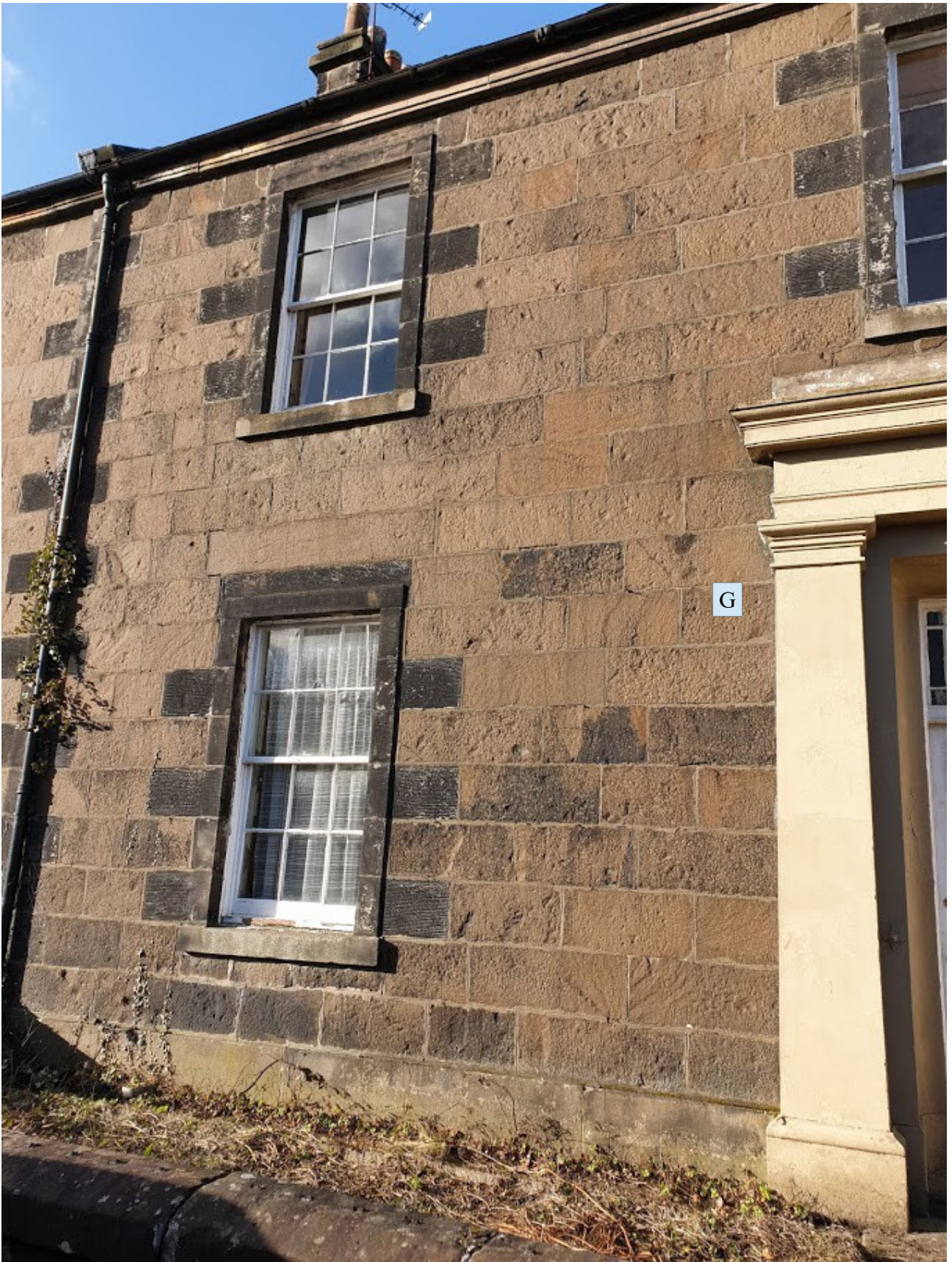
LOUNGE WINDOW TO FRONT – EXISTING TIMBER SASH AND CASE WINDOW REFURBISHED EXTRACTOR FAN GRILL FITTED FOR KITCHEN
