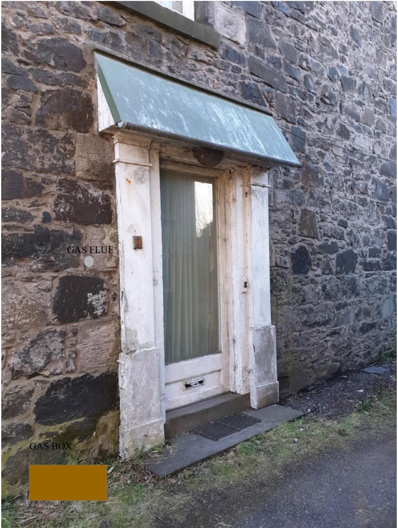
FRONT ENTRANCE DOOR INTO LOWER GROUND FLOOR FLAT – NEW COMPOSITE FRONT DOOR FITTED. NEW LIGHT FITTED. TIMBER SURROUND REPAIRED AND METAL ROOF PAINTED. BROWN GROUND MOUNTED GAS BOX FITTED AND FLUE
