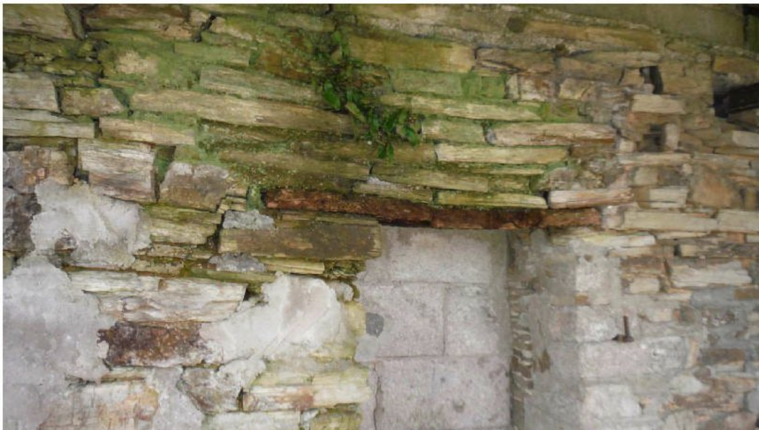
Photograph 4 Bow in the lintel over the window opening to the East Elevation
