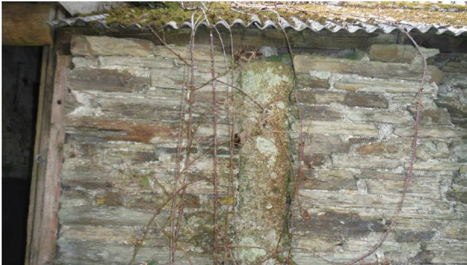
Photograph 3 Granite post with the stonework butted up to it within the east elevation wall
