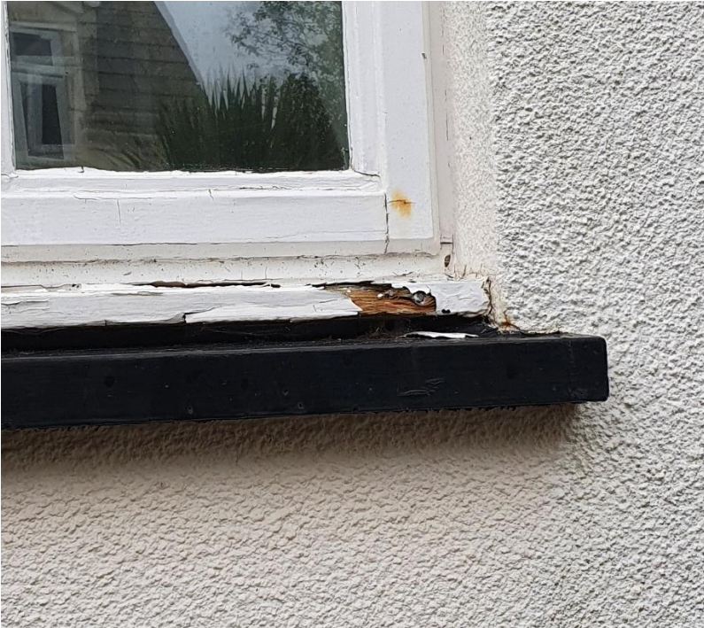
Cill rotten and casement joint defective and repaired
