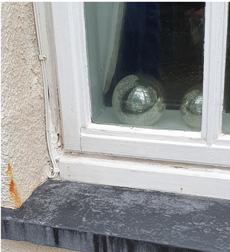
Cill rotted away and timber planted on, Frame, casement and beading rotten.
