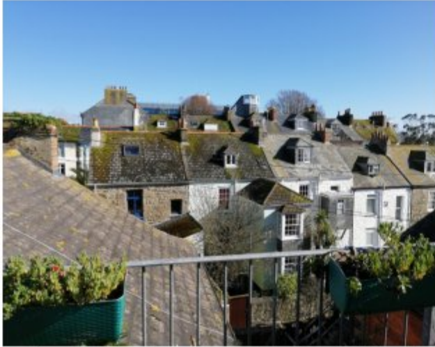
Looking East from Morrab Road to Morrab Place at nos 1-7 in front & 12 -17 behind. Showing the dry laid natural slate or cement fibre roofs.
