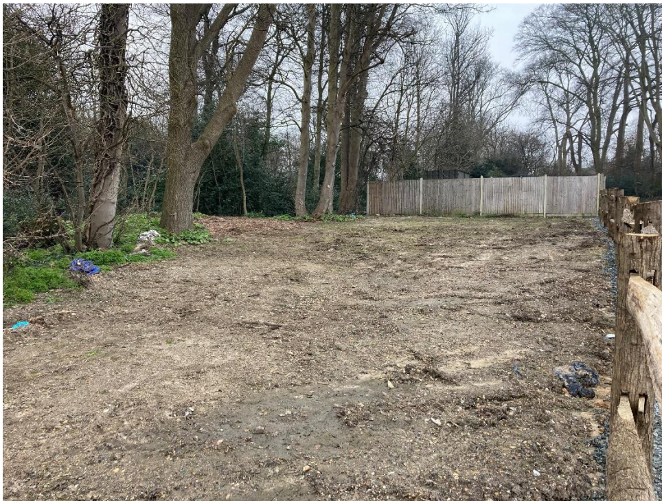
Plate 6. Minimal grading observed for in vicinity of Car Park CSA. Facing east.
