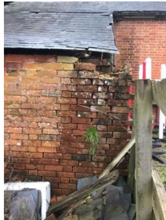
Photo 12: Gaps within the brickwork
