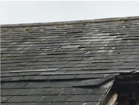
Photo 11: Raised or slipped tiles
