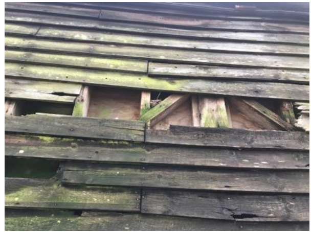
Photo 10: Holes and gaps within weatherboarding
