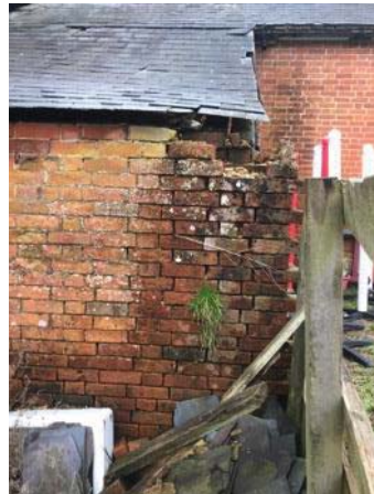
Photo 12: Gaps within the brickwork
