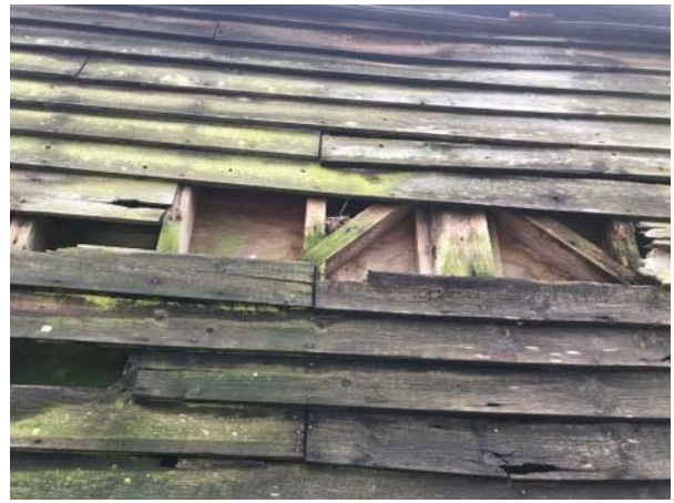
Photo 10: Holes and gaps within weatherboarding
