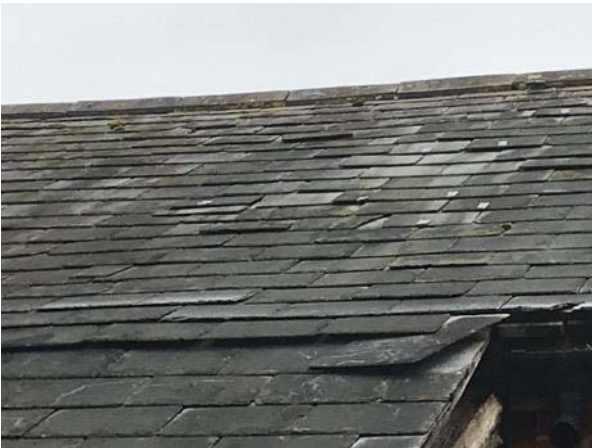
Photo 11: Raised or slipped tiles
