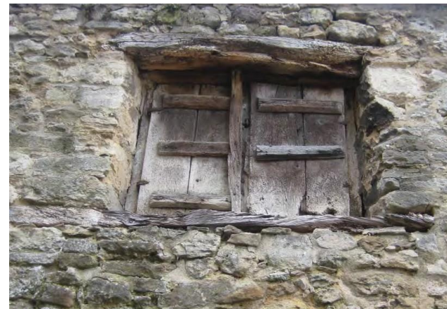
Details of features in the south wall which will all be repaired and conserve to highest conservation standards
