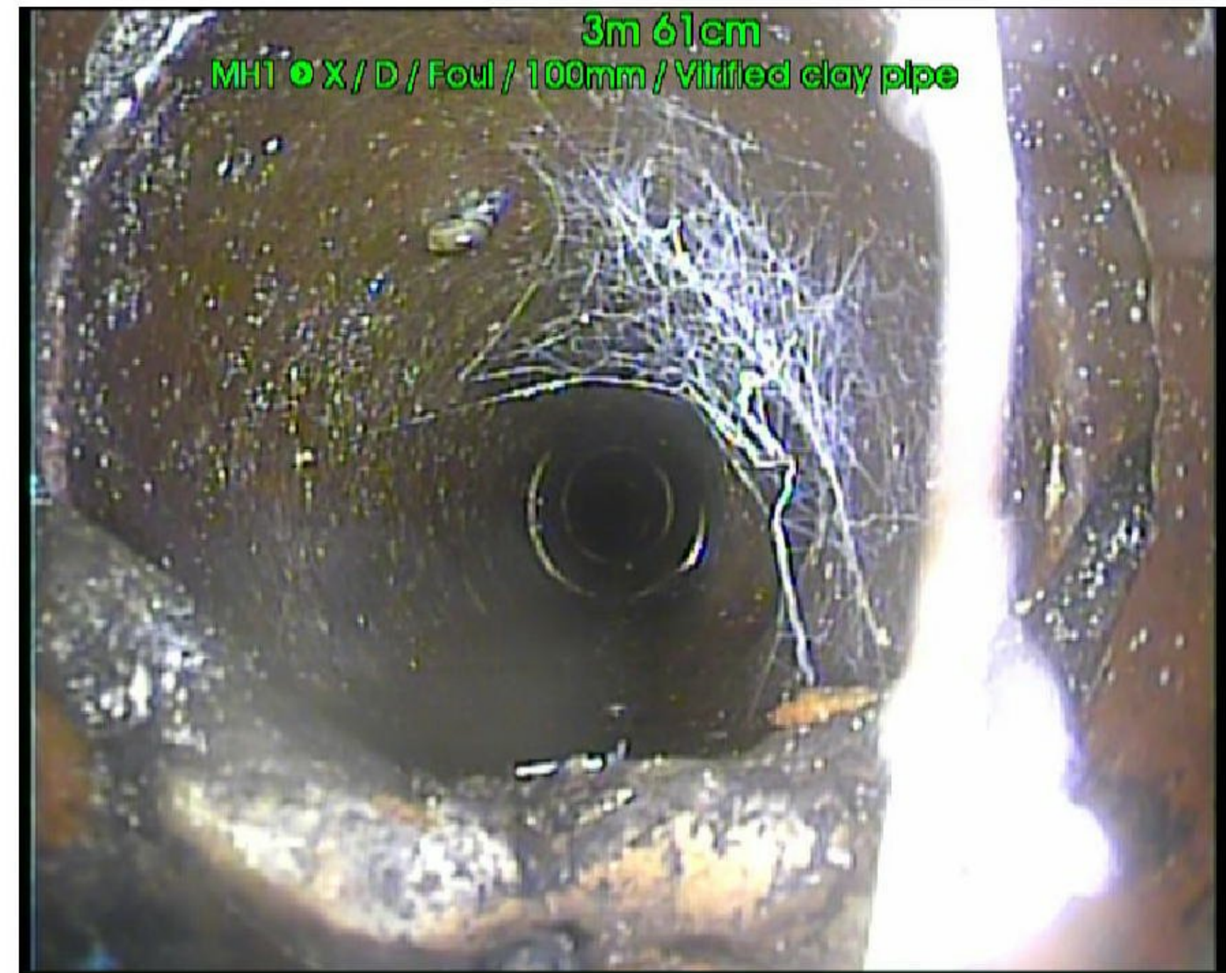
Photo: 2_2_5_A.jpg 3.61m, Attached deposits, encrustation from 4 O'Clock to 8 O'Clock 15 % cross-sectional area loss SCALE
