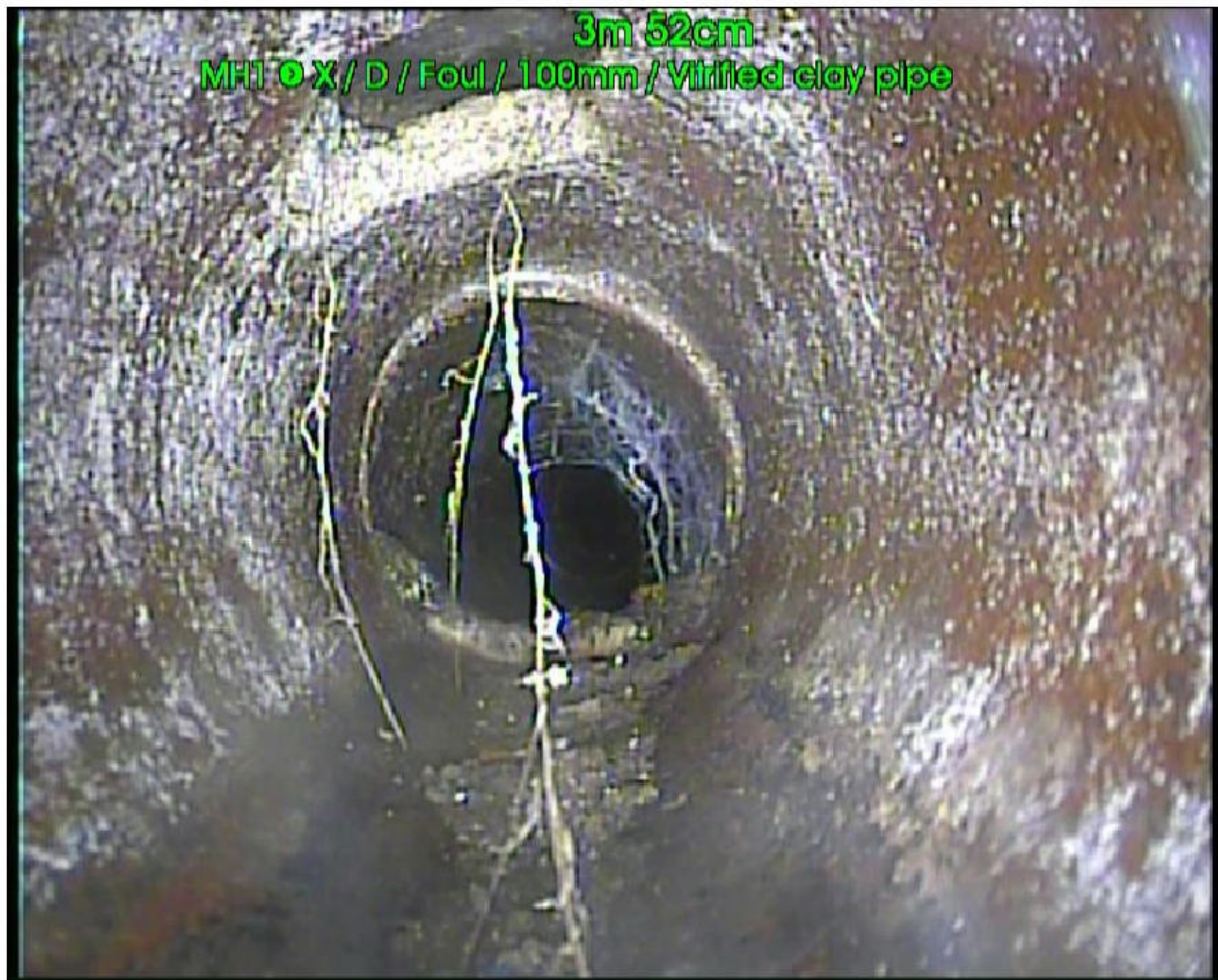
Photo: 2_2_4_A.jpg 3.52m, Hole in drain/sewer from 10 O'Clock to 11 O'Clock POSS CONNECTION FOR GULLIES
