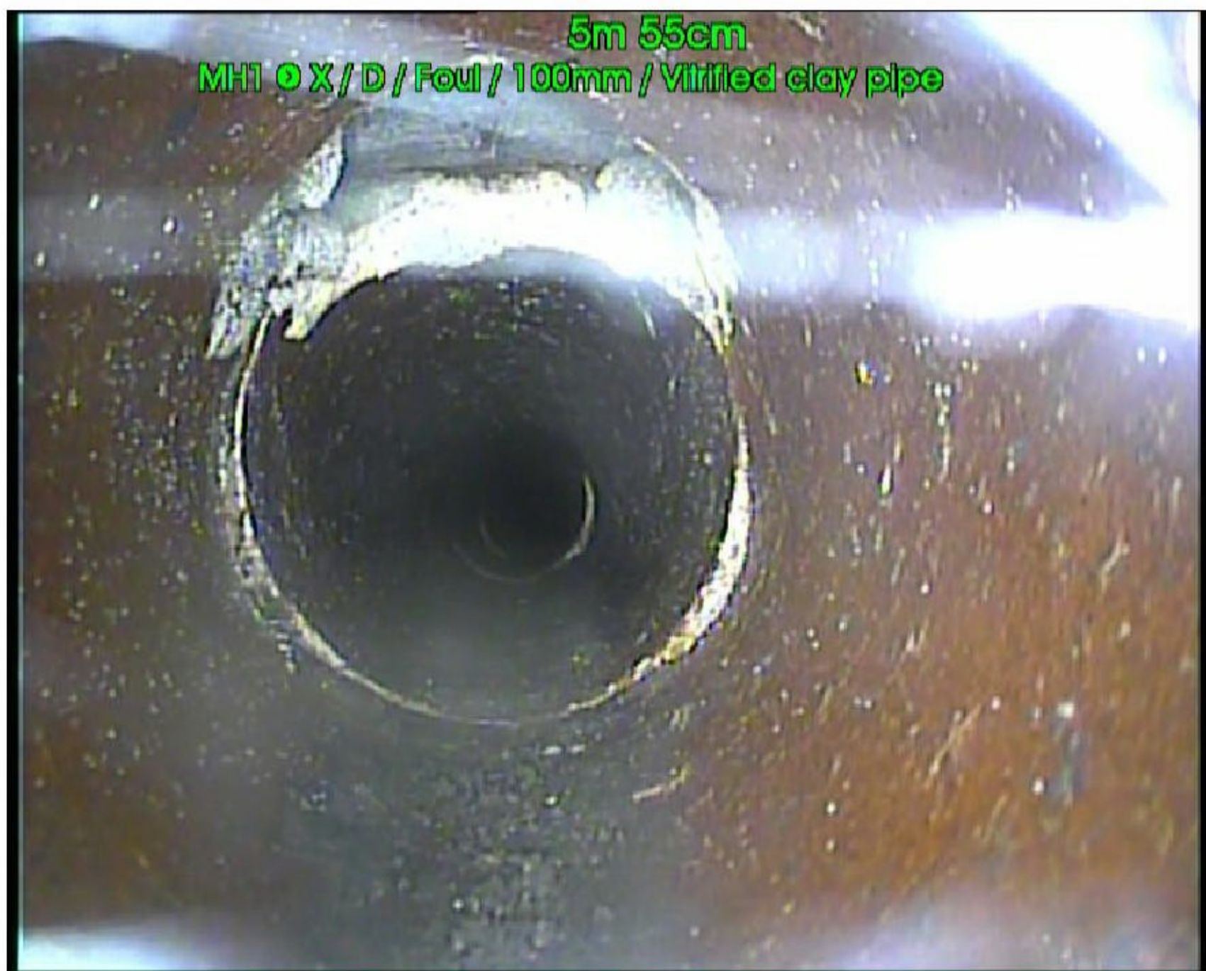
Photo: 2_2_6_A.jpg 5.55m, Hole in drain/sewer from 10 O'Clock to 2 O'Clock
