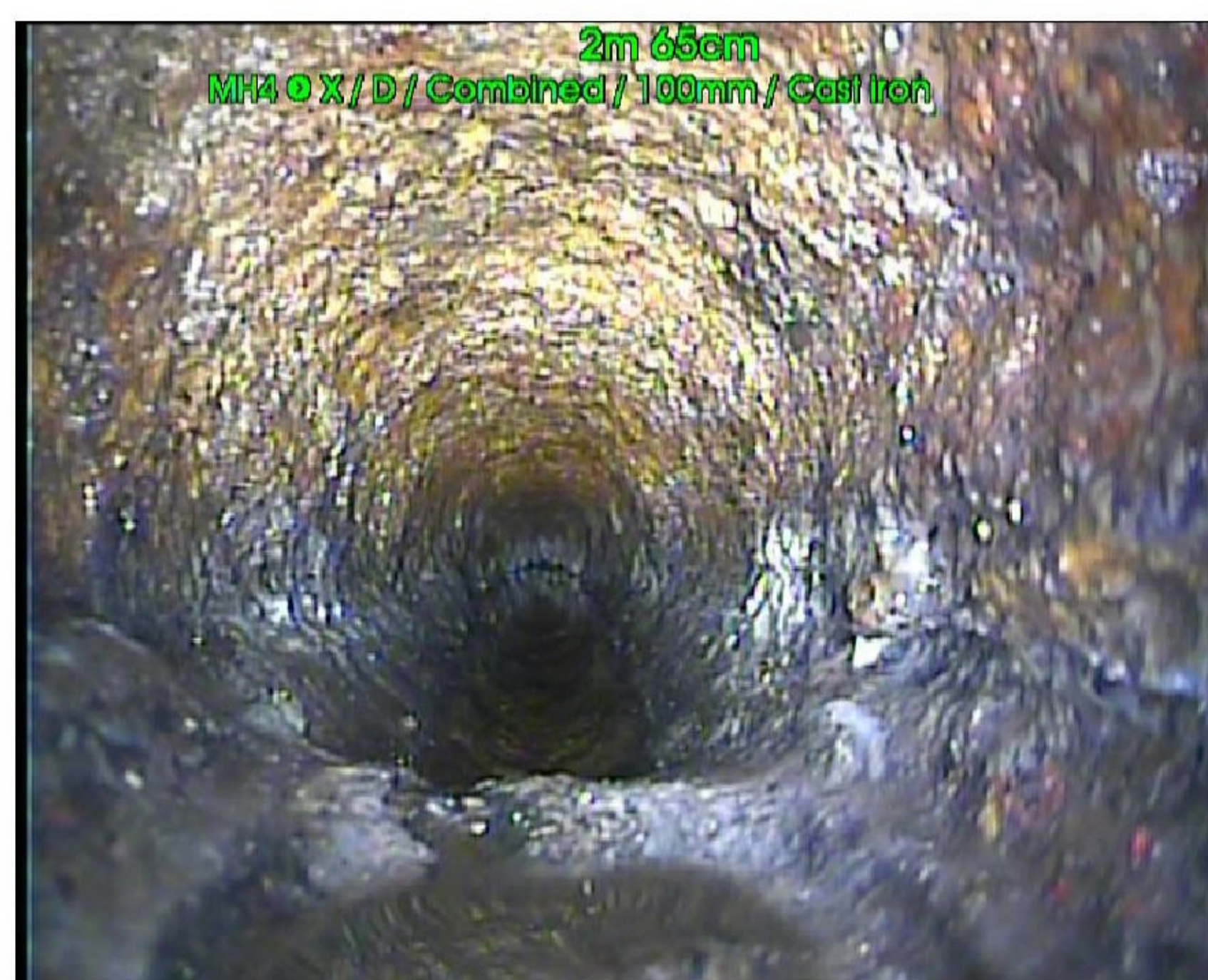
Photo: 9_9_43_A.jpg 2.6m, Attached deposits, encrustation from 5 O'Clock to 7 O'Clock 20 % cross-sectional area loss
