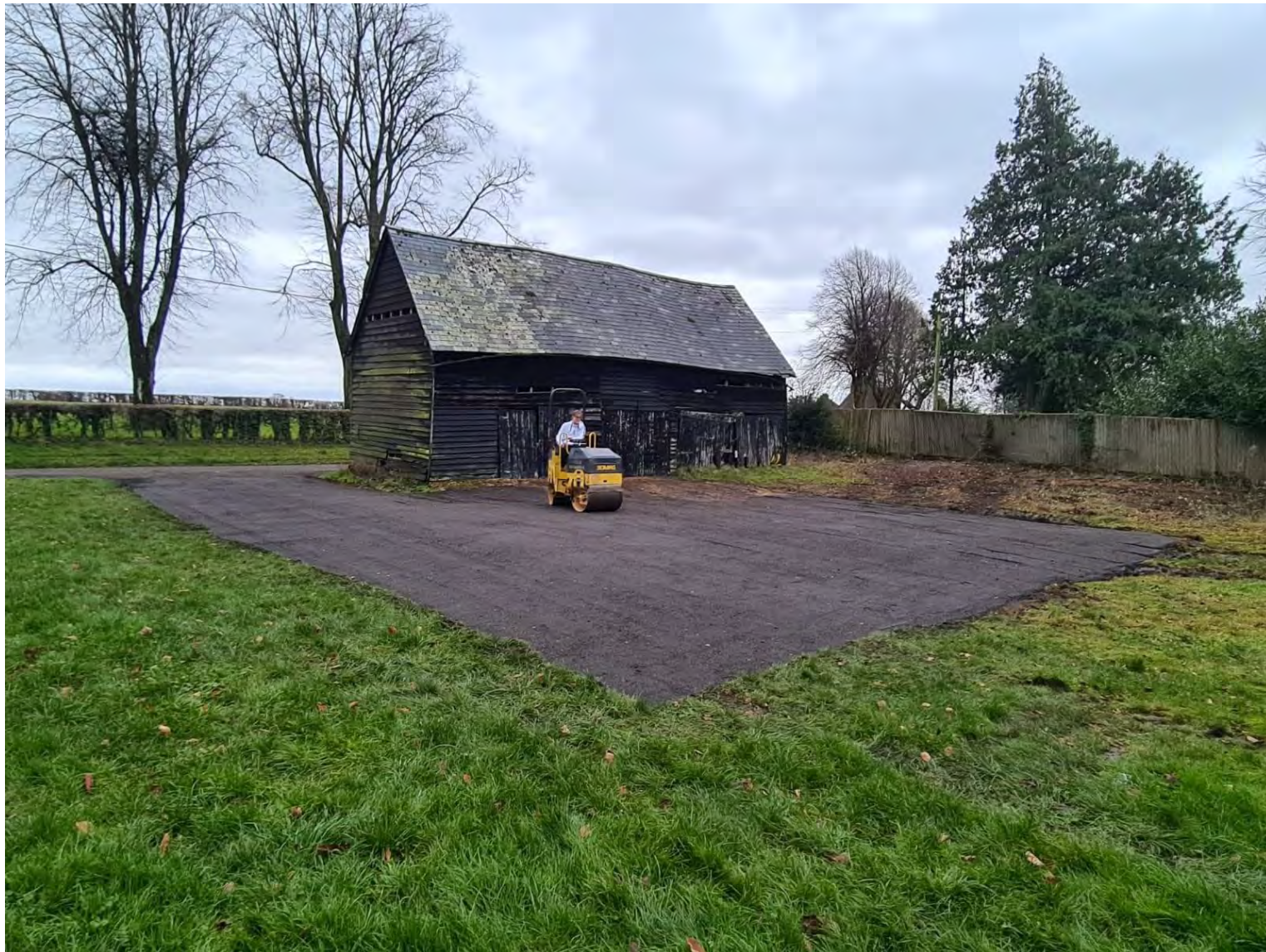
Photographs . The Black Barn Access and Parking Area . 11st and 12th January 2021
