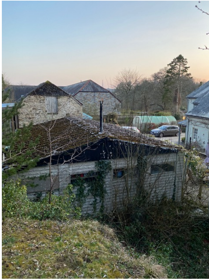
Photo of garage from the North side with the barn and the housing development (2006) beyond
