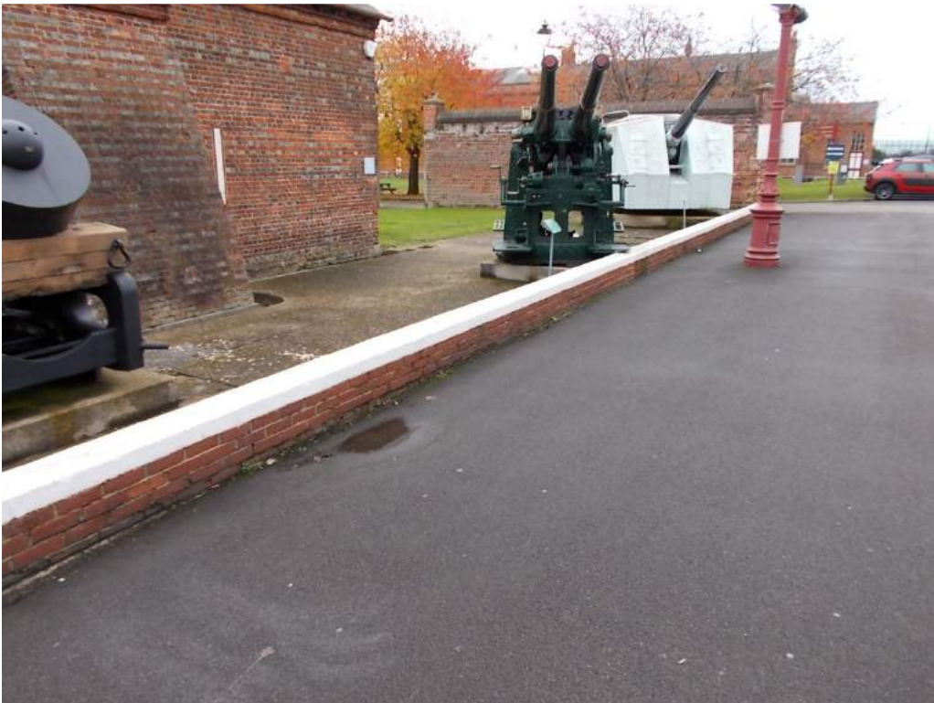
Existing wall within Explosion Museum with potential to act as internal flood wall
