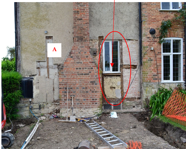
Fig 6: Detail of the ground floor of the east gable in 2011 Right photo
