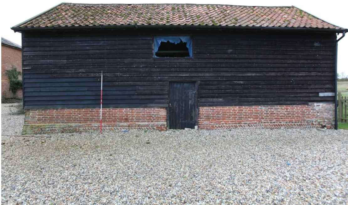
Illus. 6. The northern elevation showing its renewed 20th century cladding of stained pine boards and the original central door respected by the brick plinth which is laid in Monk Bond. The first-floor windows in both this and the southern elevations appear to be later insertions.
