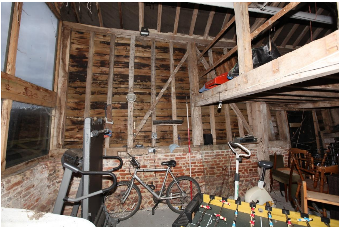
Illus. 10. The northern internal wall of bay D from which the original ceiling joists have been removed showing the rebuilt western gable on the left. The left-hand stud and sections of the roof-plate and sill have also been renewed but the brick plinth is original to the building. The diagonal braces are nailed to the principal posts, which lack jowls in the typical manner of the mid-19 th century, and many studs show evidence of re-use from an 18 th or early-19 th century structure.
