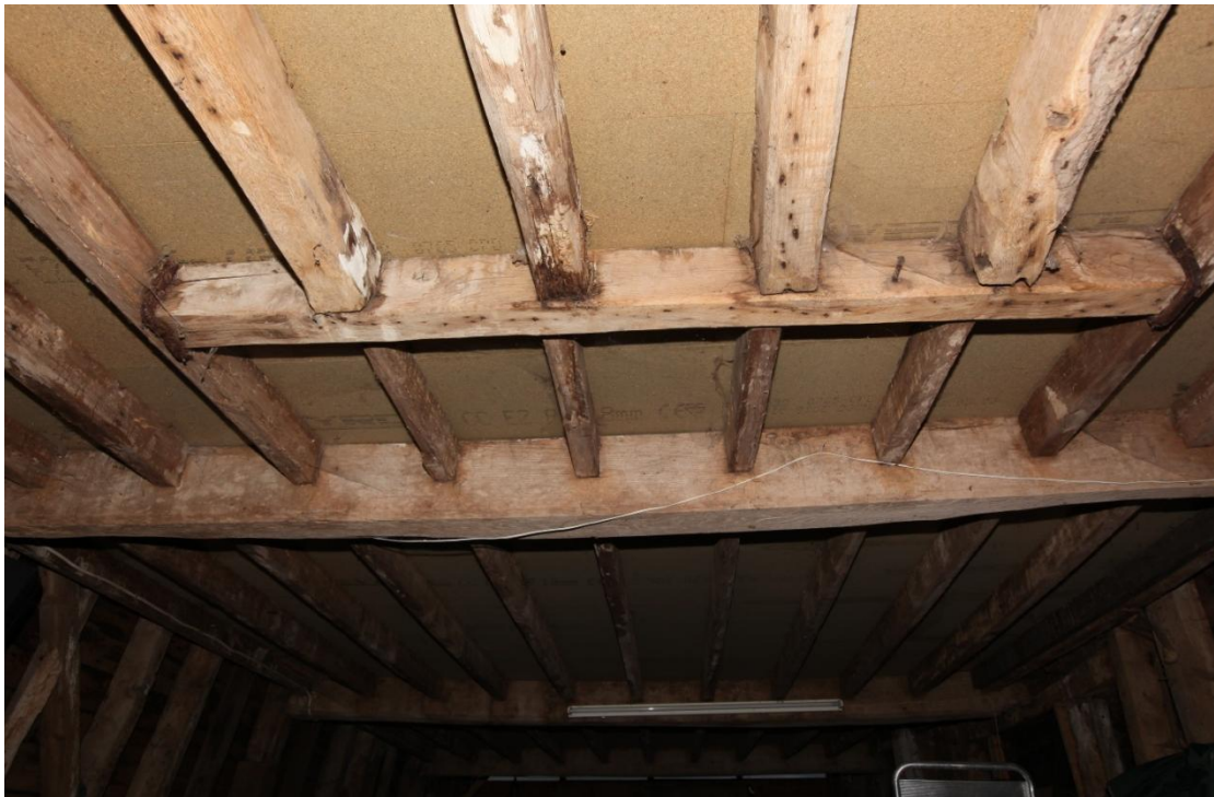
Illus. 8. The ground-floor ceiling of bay A from the eastern gable showing the blocked trap that may have accommodated an internal stair or milling equipment. The trimmer and the joists in the foreground differ from the plain pine joists elsewhere in the ceiling and bear evidence of lath-and-plaster having been re-used from elsewhere.
