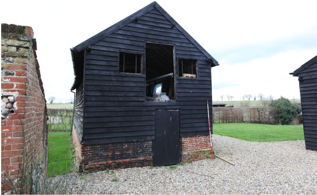
Illus. 5. The eastern external gable showing the loading door to the loft which is offset on the right suggesting an external stair once rose from the left. The ground-floor entrance is respected by closers (quarter-bricks) in the brick plinth and is therefore an original feature.
