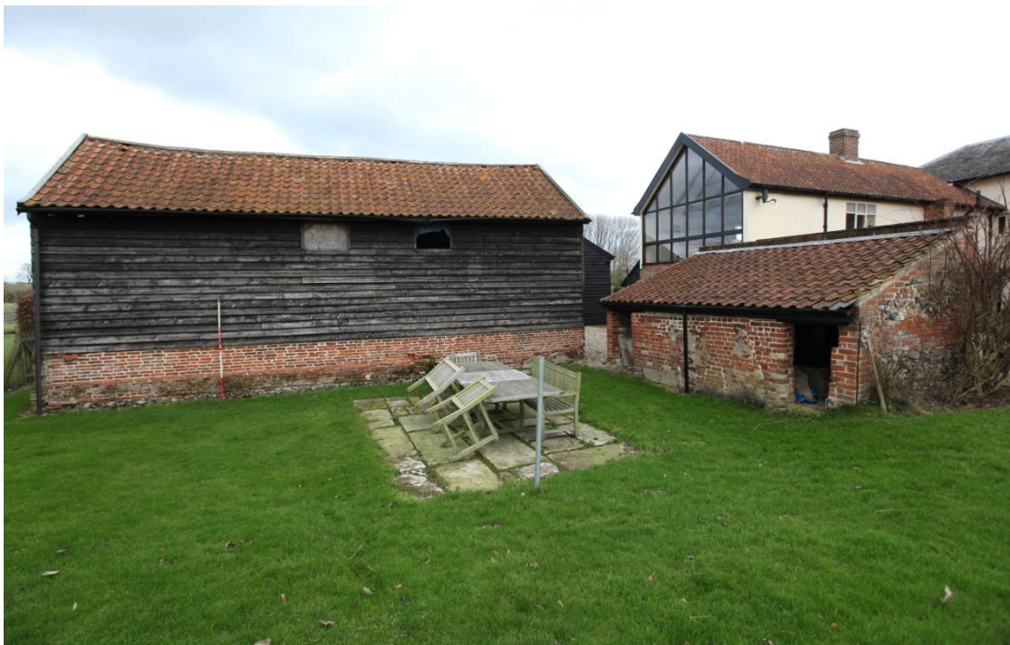
Illus. 4. The rear barn's southern elevation showing its close proximity to the much altered 19 th century range of pig sties on the right, which preserves the outlines of two earlier arched apertures between its existing entrances. The two buildings almost adjoin corner-to-corner as on the Ordnance Survey of 1883 but in marked contrast to the situation shown in 1837 when a building on the site of the rear barn extended much further to the right.
