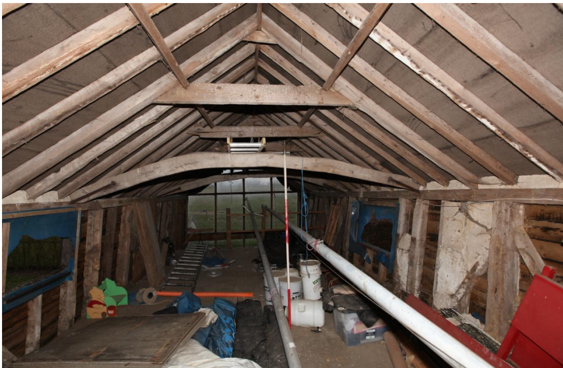
Illus. 14. The loft from the eastern gable showing its ostensibly original clasped-purlin roof with a ridge board, purlins and nailed collars of pine. The two tie-beams, which are cambered to increase headroom, are also of pine and are secured to the roof-plates with original iron straps. A section of original infill of rendered brick is visible on the right and many rafters show signs of re-use with the remains of lath-and-plaster that are not relevant to the existing building.
