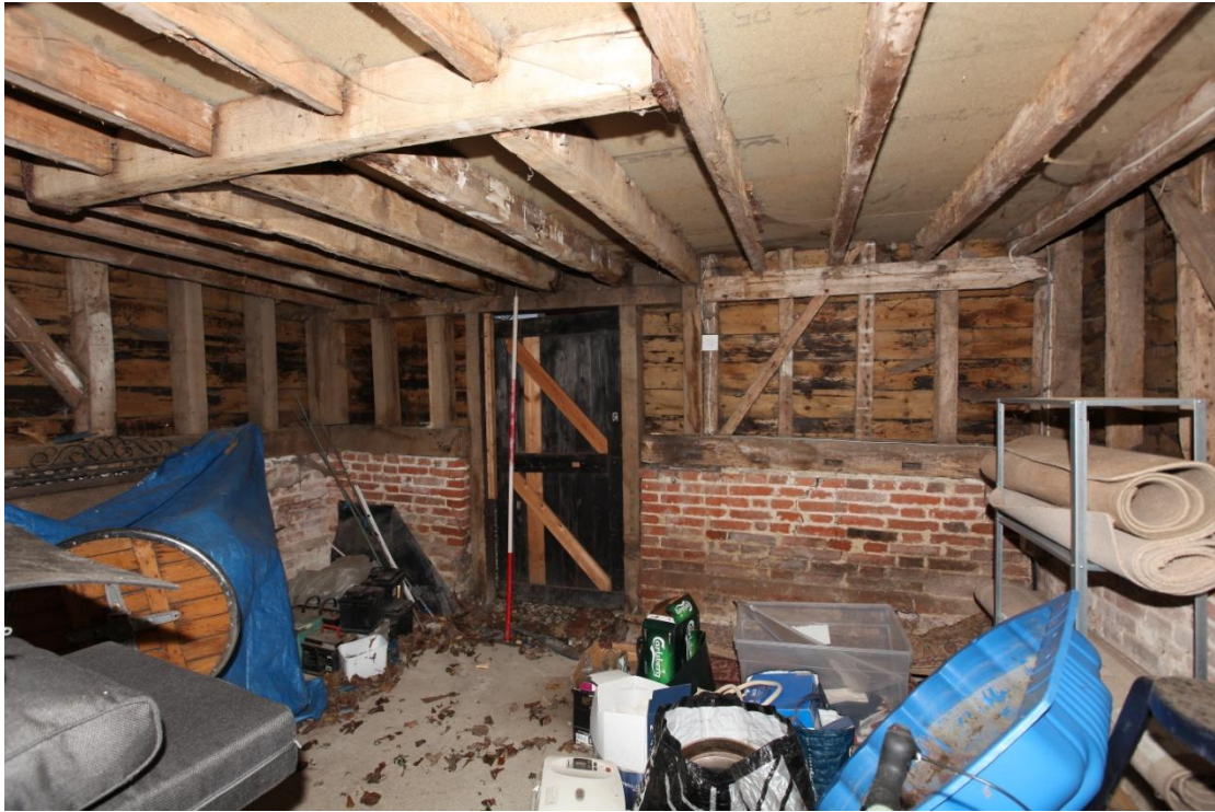
Illus. 7. The internal eastern gable showing the original studwork to the right of the door with a narrow diagonal primary brace and evidence of re-used timber (as some studs bear the scars of lath-and-plaster while others do not). The studs and sill to the left of the door were renewed in the late-20 th century.
