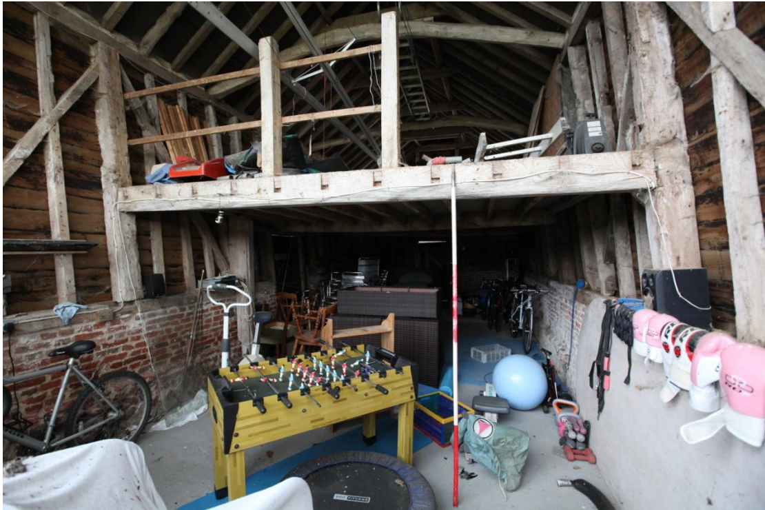
Illus. 11. The interior looking east from the western gable showing the missing ceiling in bay D with empty joist mortises in the binding joist. The two posts above may have secured a piece of milling machinery.
