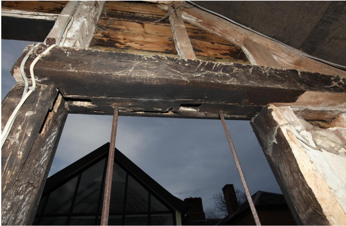
Illus. 13. A detail of the underside of the pine tie-beam in the eastern gable showing empty stud mortises that suggest both the window and door are later insertions – or that the timber has been re-used. A small circular mortise in the centre housed a wooden mullion between the surviving iron bars.
