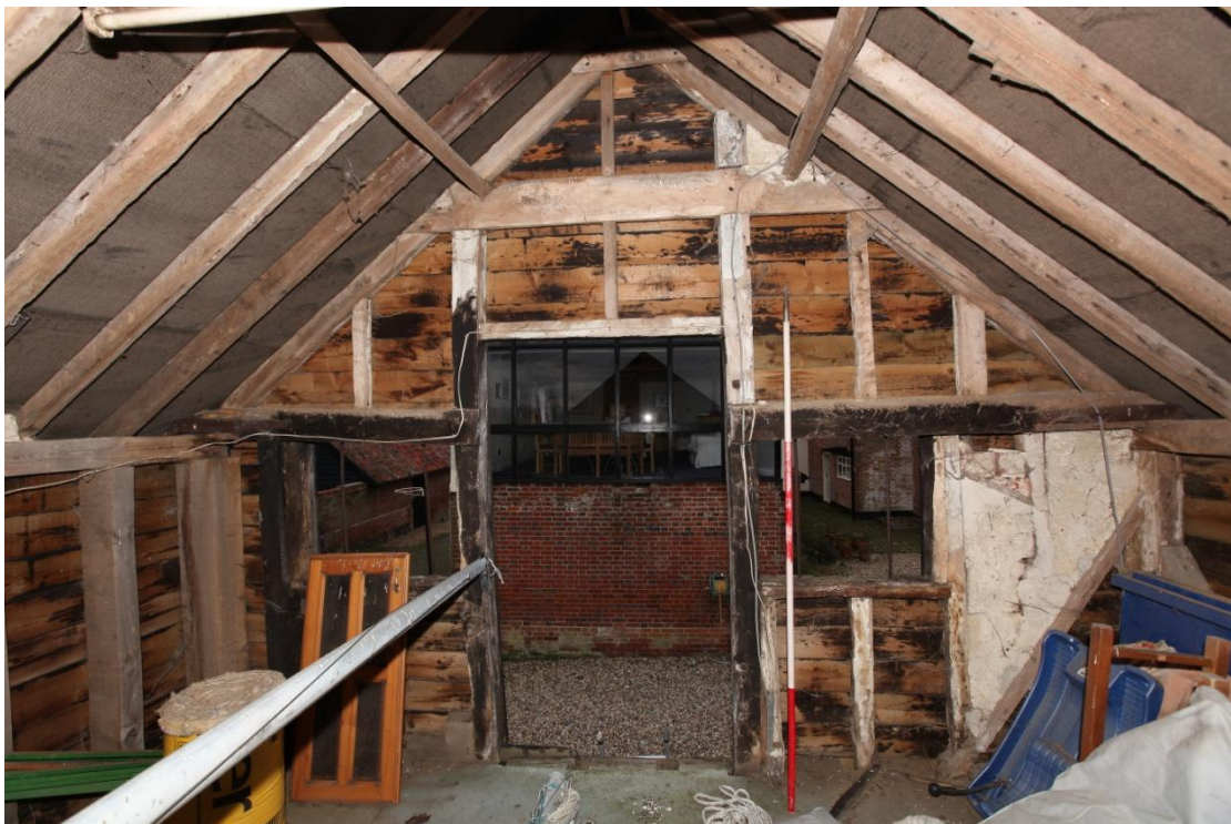
Illus. 12. The eastern internal gable of the loft showing the loading door slightly to the left of centre with an intact section of original rendered brick infill on the right. The post and stud of the northern elevation on the left are modern replacements.
