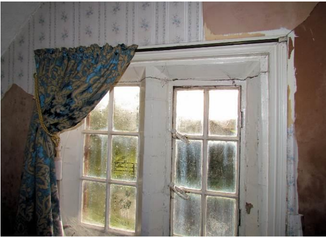
Crack Across Terracotta Window Surround at South End, First Floor
