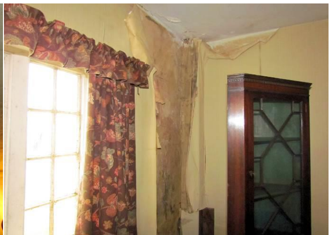
Peeling Wallpaper in Central Room
