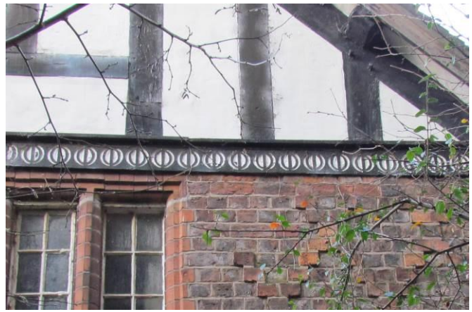
Moulding on Tie-beam
