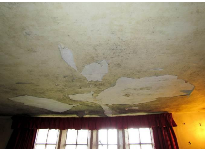
Mould and Peeling Paint in Cross-wing
