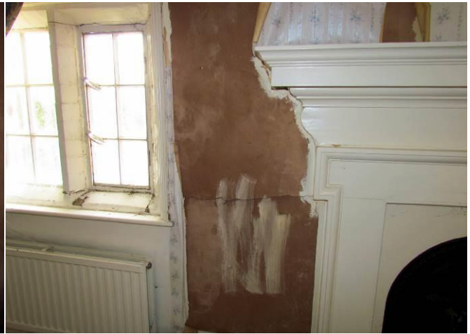
Crack in Plaster at South End
