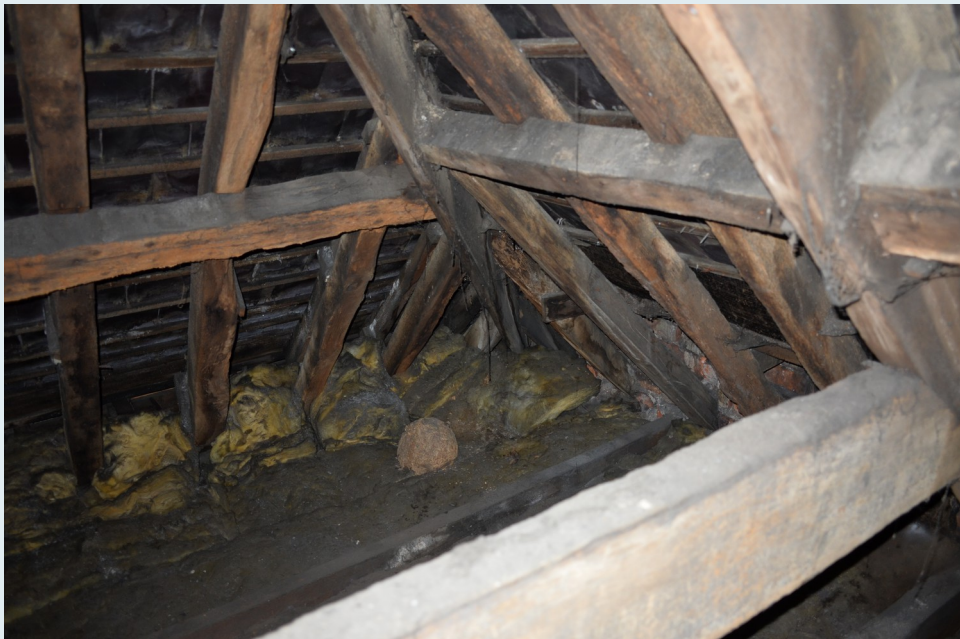
Roof structure viewed from centre of property facing front – note staining and evidence of rainwater penetration to rafters
