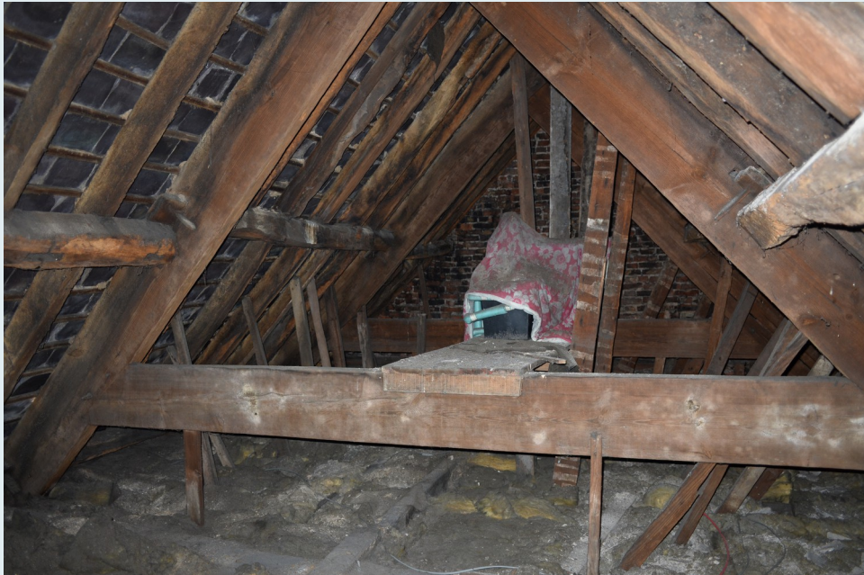
Roof structure viewed from centre of property facing rear – note redundant galvanised tanks to be removed during works
