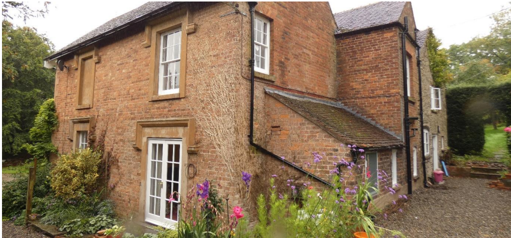
A single storey extension would have a corridor link into the french windows
