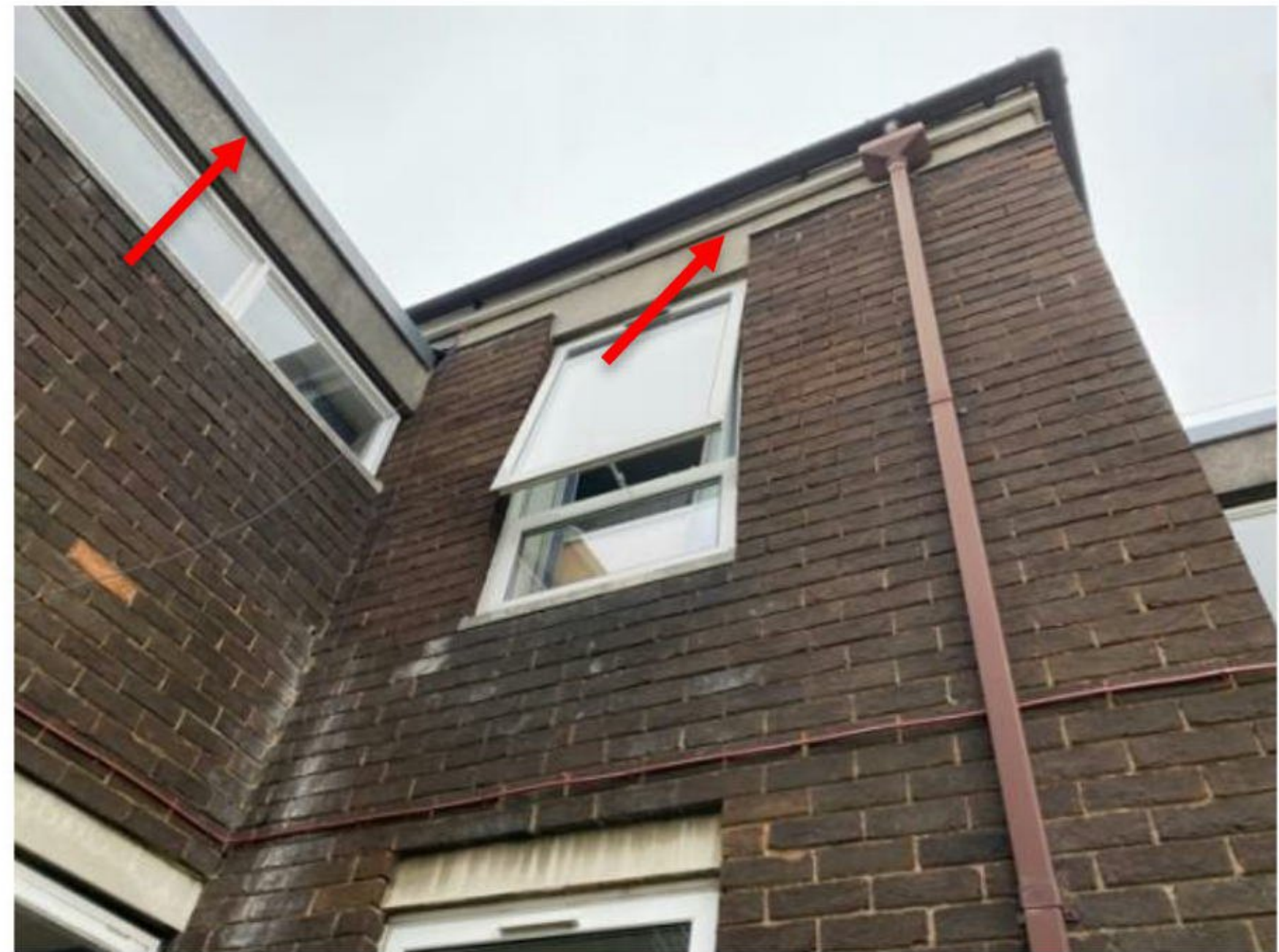
Photograph 2: Eastern elevation indicating gaps beneath rubber and fascia
