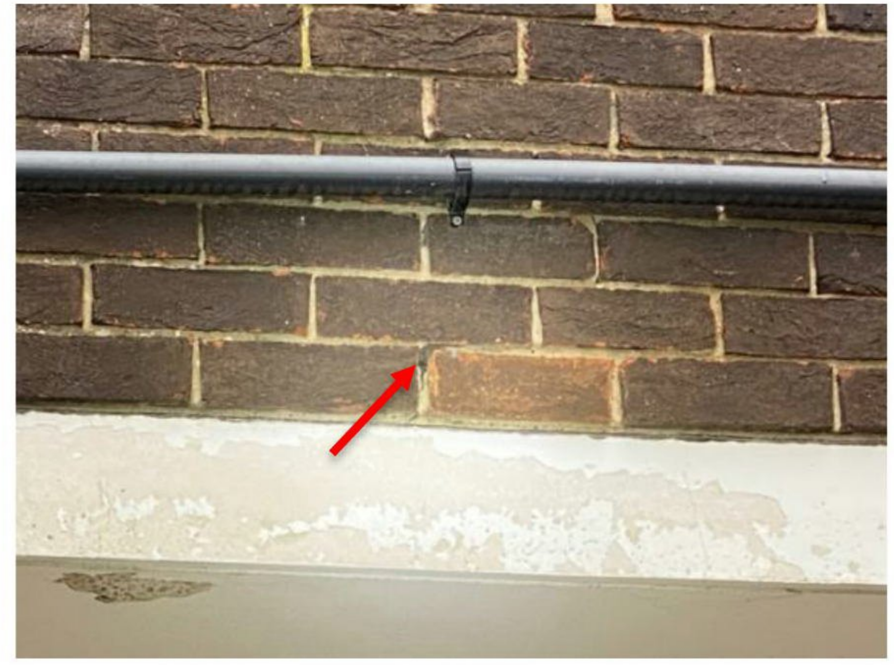
Photograph 4: Missing mortar on western aspect
