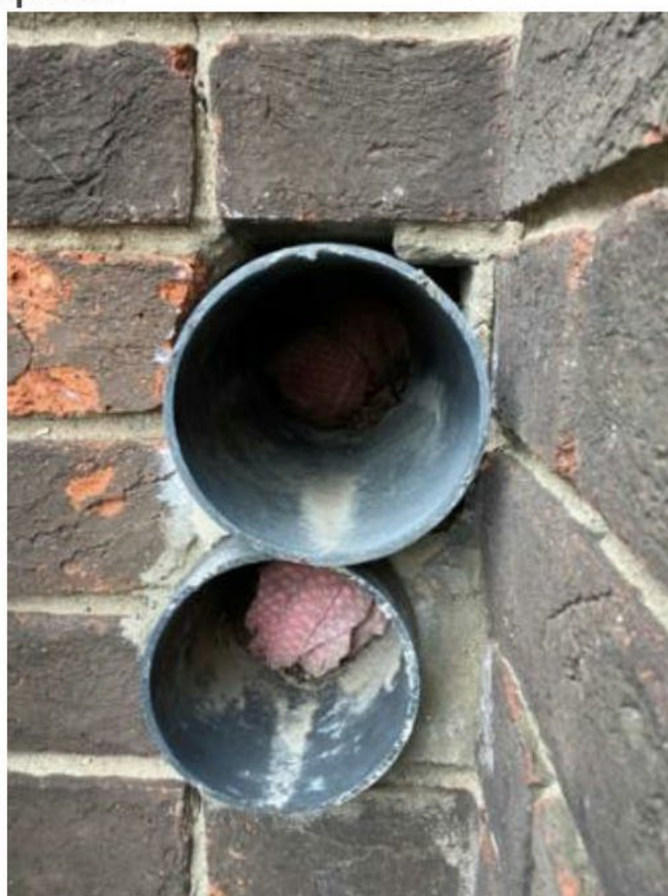
Photograph 5: Gaps around pipework on western aspect
