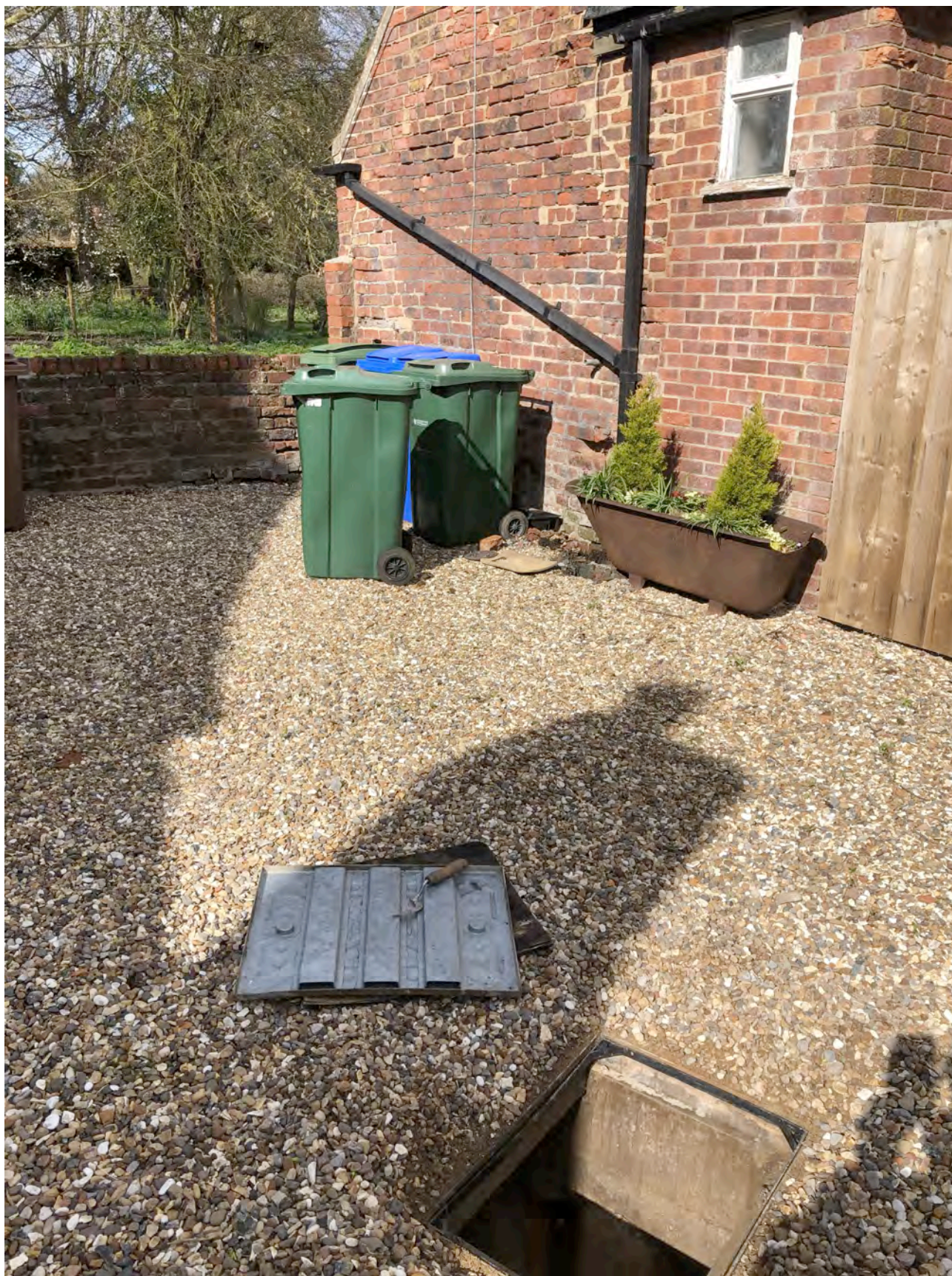
Gable end of No.21A (Application property) with rainwater downpipe visible, with Inspection chamber in the foreground.
