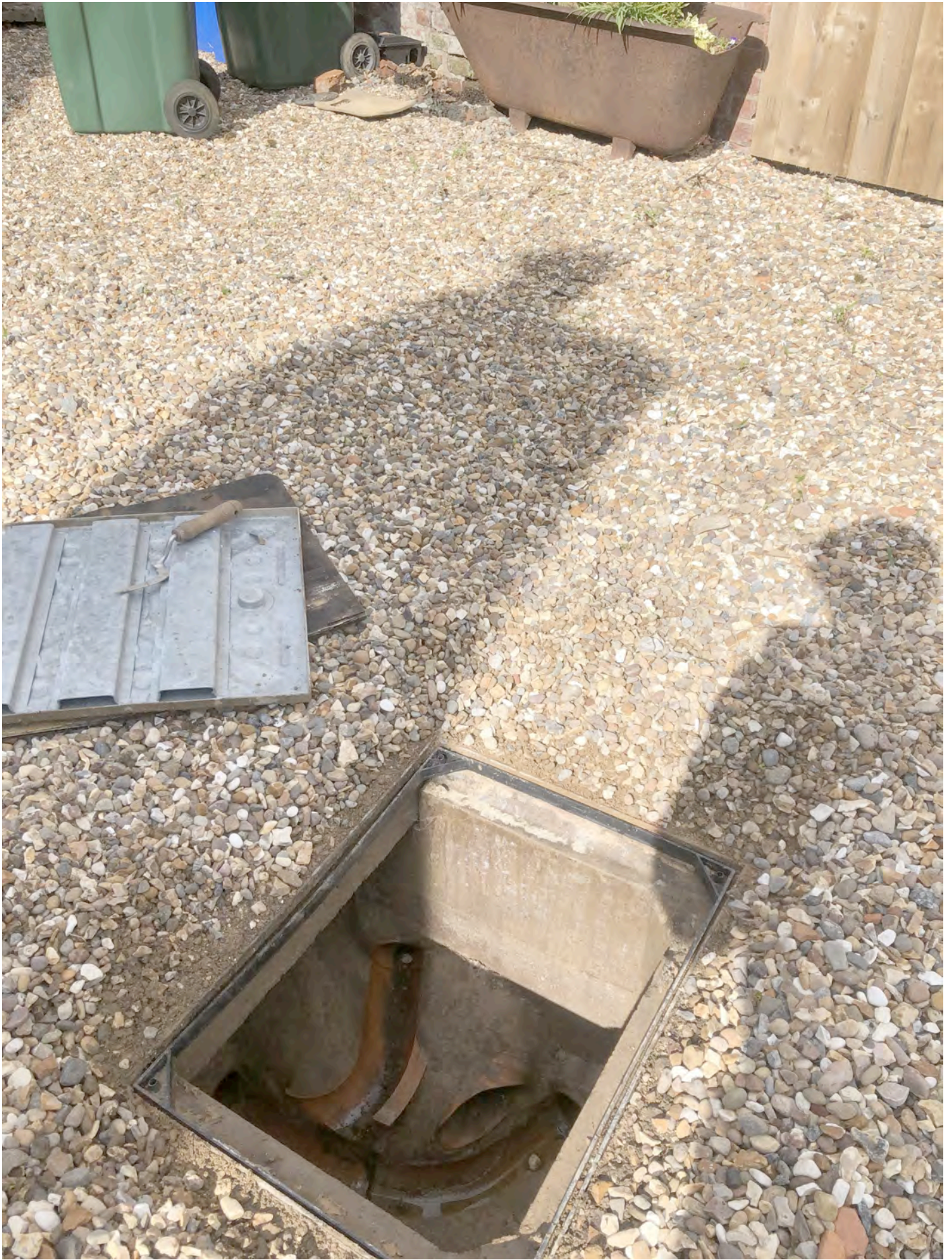
Inspection chamber, with internal arrangement visible
