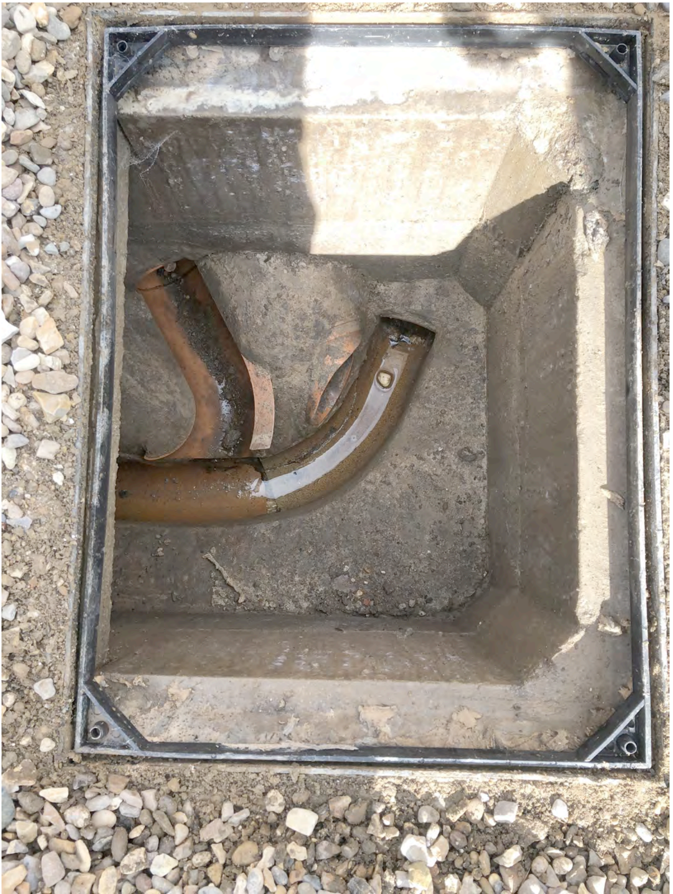
The inspection chamber receives: (L to R): Rainwater from No.21A gable; foul from No.21A; foul from No.21. There is then the single discharge pipe to the main sewer under Eastgate.
