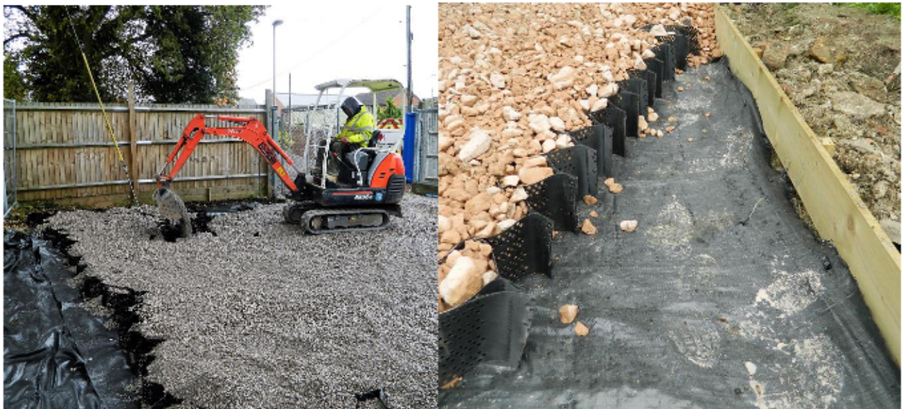
Figure 5. Photographs illustrating cellular confinement system used to form an above-ground no-dig surface.
