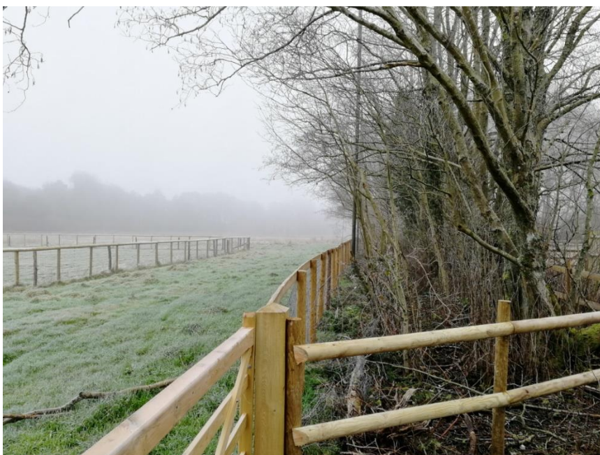
Figure 3. Photograph confirming that fencing has been erected adjacent to G2 and will delineate a construction exclusion zone.
