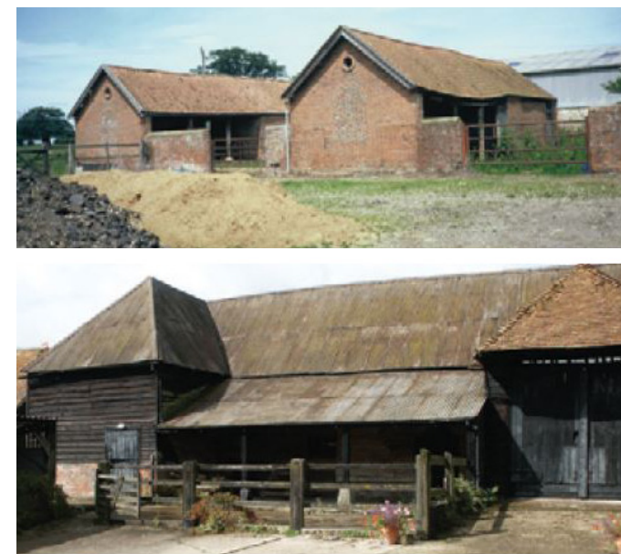
Various roof forms and interesting solid / void creates attractive building typology suitable for a range of uses.
