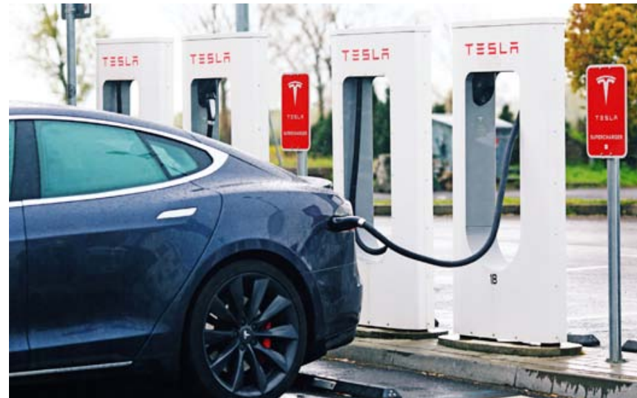
Electric car charging point
