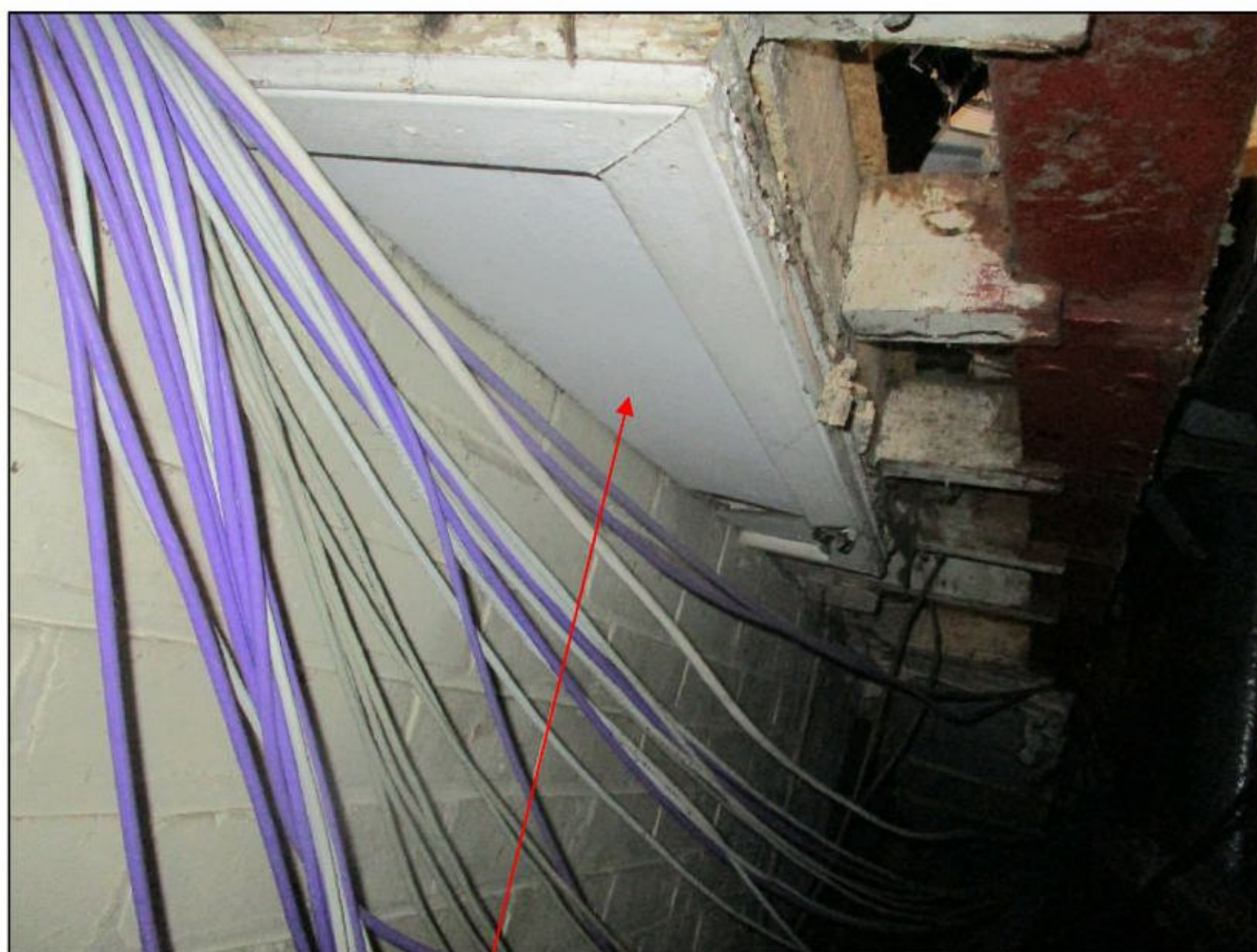
UNABLE TO ACCESS BEYOND WALL – 2m2 AS SEEN ONLY
