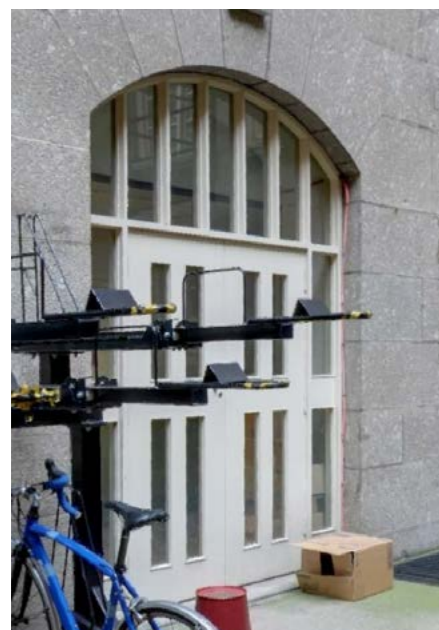
1970's doors to be removed
