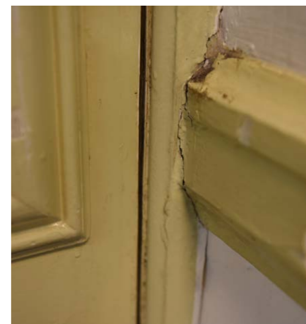
Example of existing damaged joinery item to be repaired
