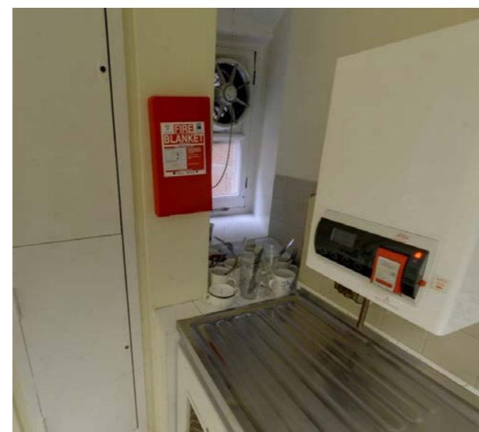
Existing tea point with local extract fan mounted in courtyard facing window
