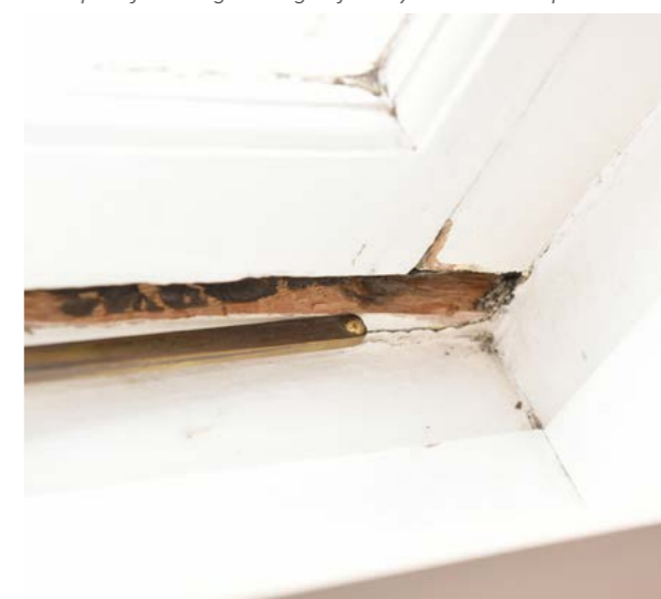
Example of existing damaged joinery item to be repaired
