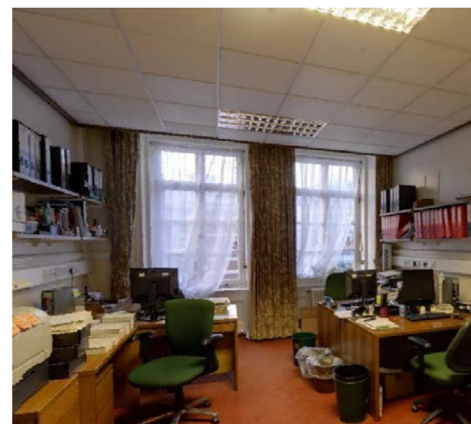
Example of office space with suspended grid ceiling, radiators beneath windows and surface mounted services trunking on the walls. Windows currently restricted opening and single glazed.
