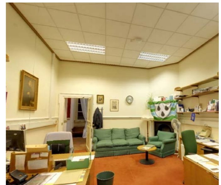
Current office illustrating piecemeal modifications to services including suspended grid ceilings, mid level surface mounted trunking and renewed decoration. Note impact of trunking on dado rail.
