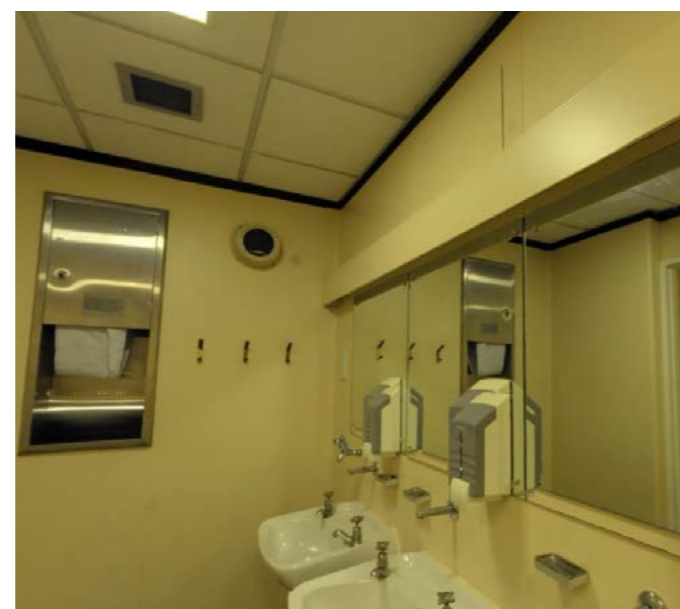
Existing WC with minimal servicing and no heating.
