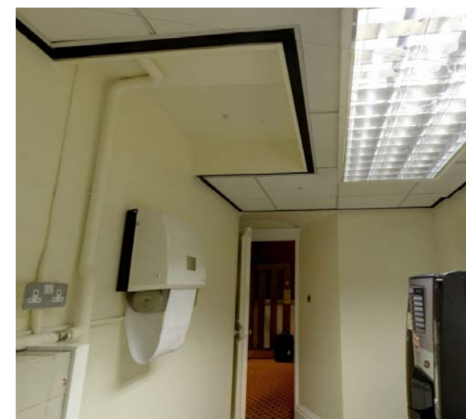
Existing pipework exposed with insulation damaged and worn out
