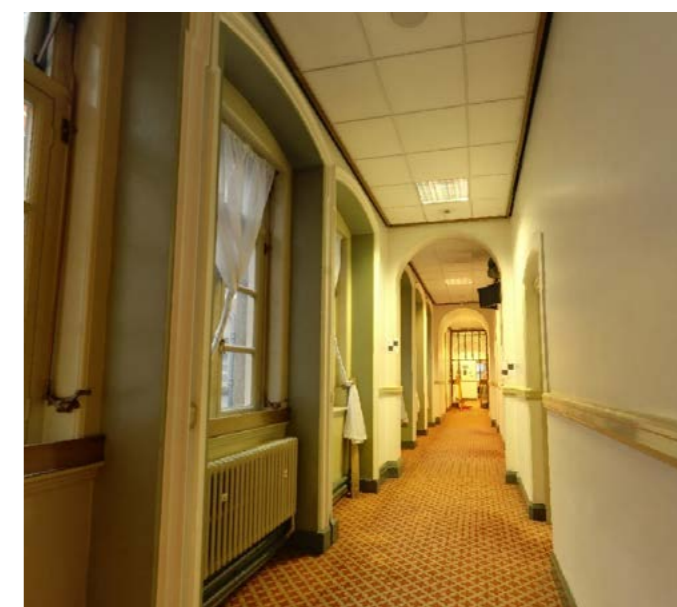
Example of corridor space with suspended grid ceiling, radiators beneath windows and timber cross corridor screens.
