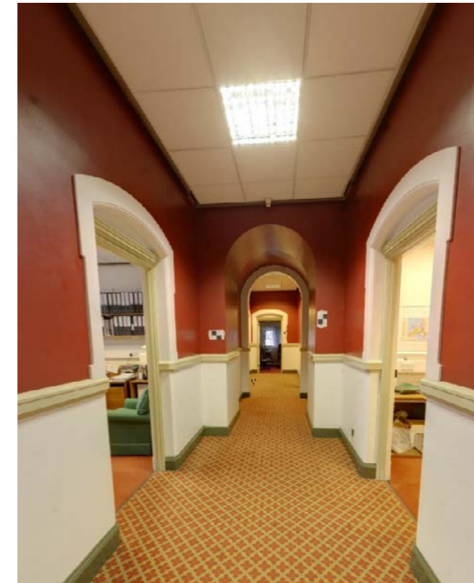
Low inserted ceilings to corridors clash with vaulted ceilings
