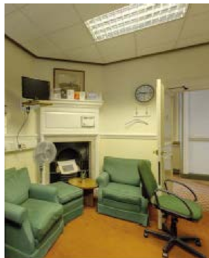
Lay-in ceiling grid clashes with layout of office/fireplace
