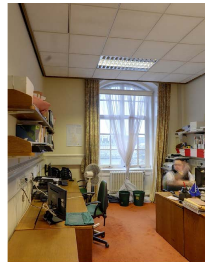
Low inserted ceilings to offices interfere with view of windows
