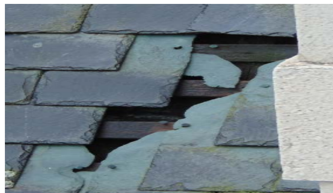
Hole in slate covering to NSN roof
