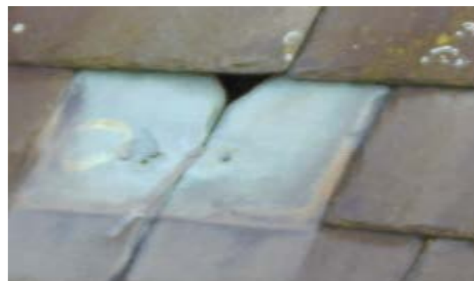
Series of missing slates on NSN roof
