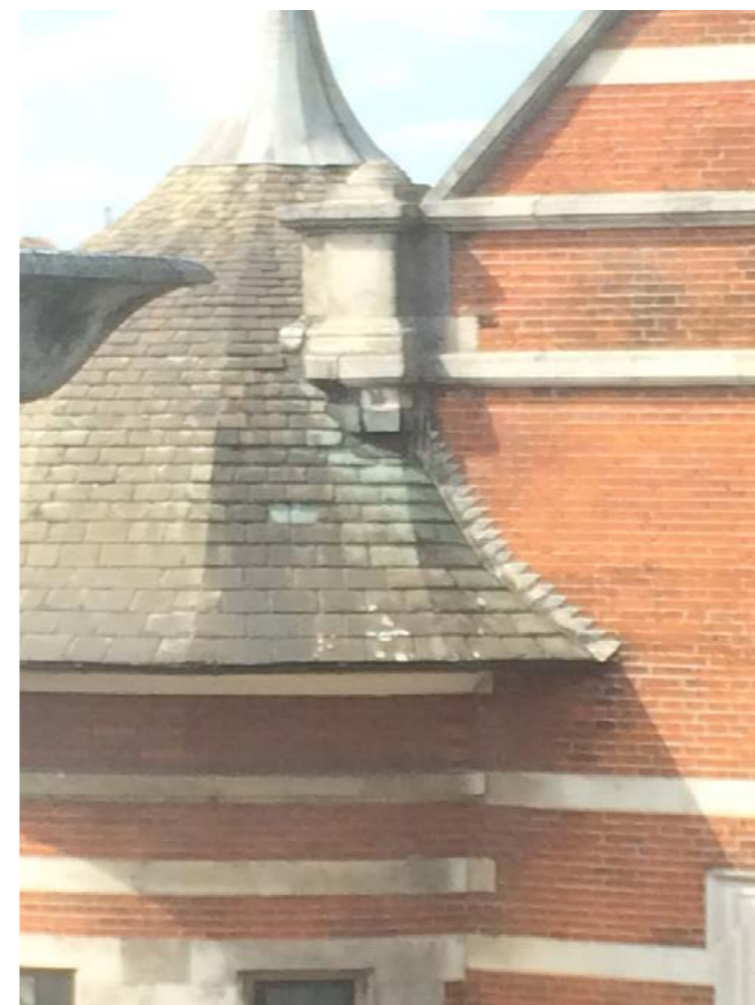
Photographic survey of south elevation south west turret shows missing and lifting slates
