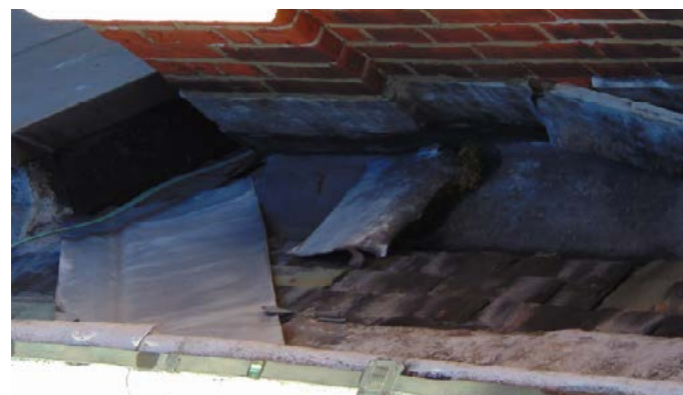
Slates slipped down to lower areas of NSN roof
