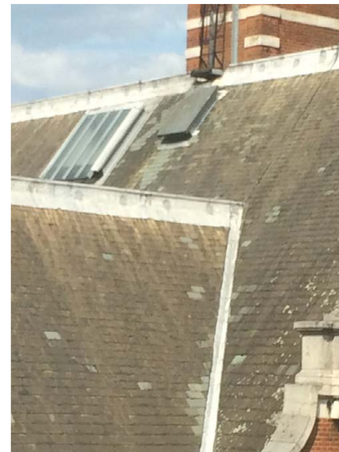
Photographic survey of south elevation shows various missing slates
