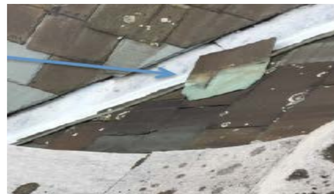
Slipped slates in NSN gutters
