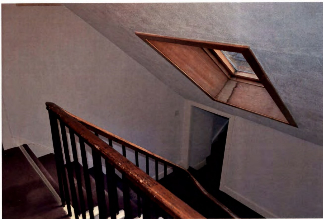
Photo of Existing Stair Link opening [ to be infilled] and present large stairwell velux rooflight.
