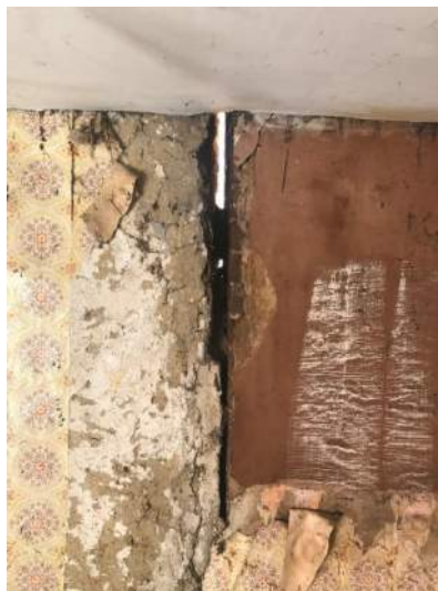
Fig 8 – Internal view of separation of clay lump gable end wall away from central brick chimney, with daylight clearly visible through significant cracking
