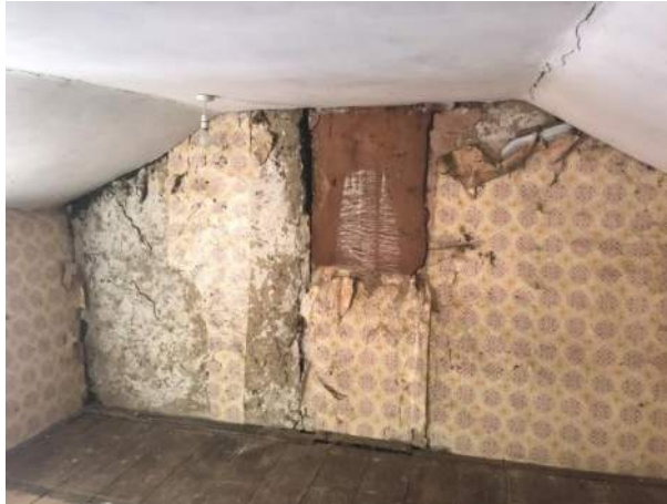
Fig 7 – Internal view of clay lump gable end wall with central brick chimney, also showing cracking due to spreading of roof structure and outwards leaning side walls
