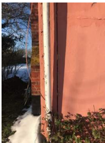
Fig 10 – Close-up of full height crack separation of clay lump gable end and side wall
