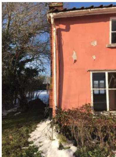
Fig 9 – External view of full height crack separation of clay lump gable end and side wall
