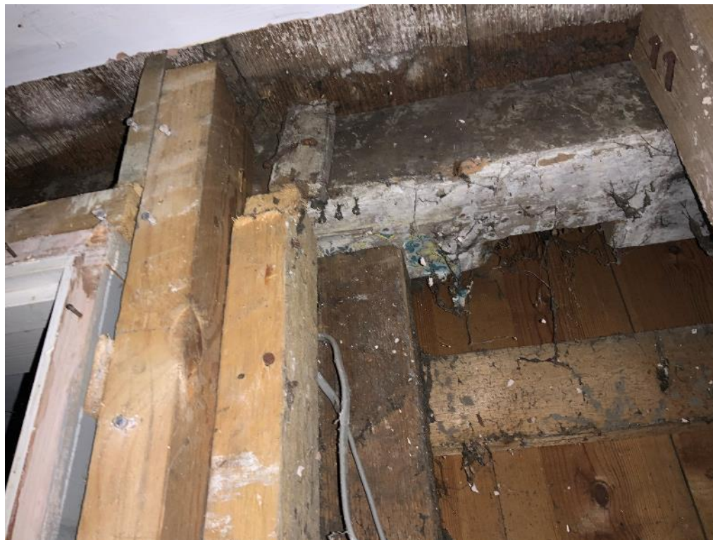
Historic floor joist with diagonal half lap joint. Historic wall paper under staircase studwork structure.
