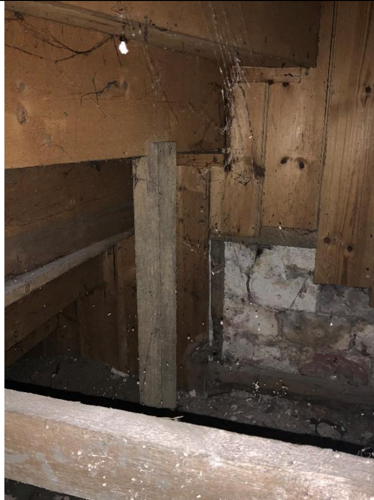
Poorly detailed panelling and general construction
