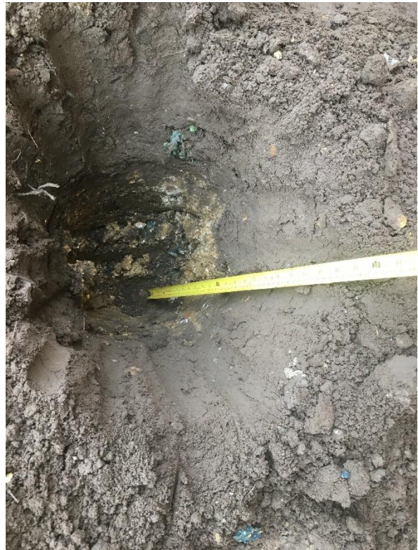
Photograph 8 , taken on the 15 th February 2021 showing HDPT31-06 following the removal of the coarse concrete gravel.
