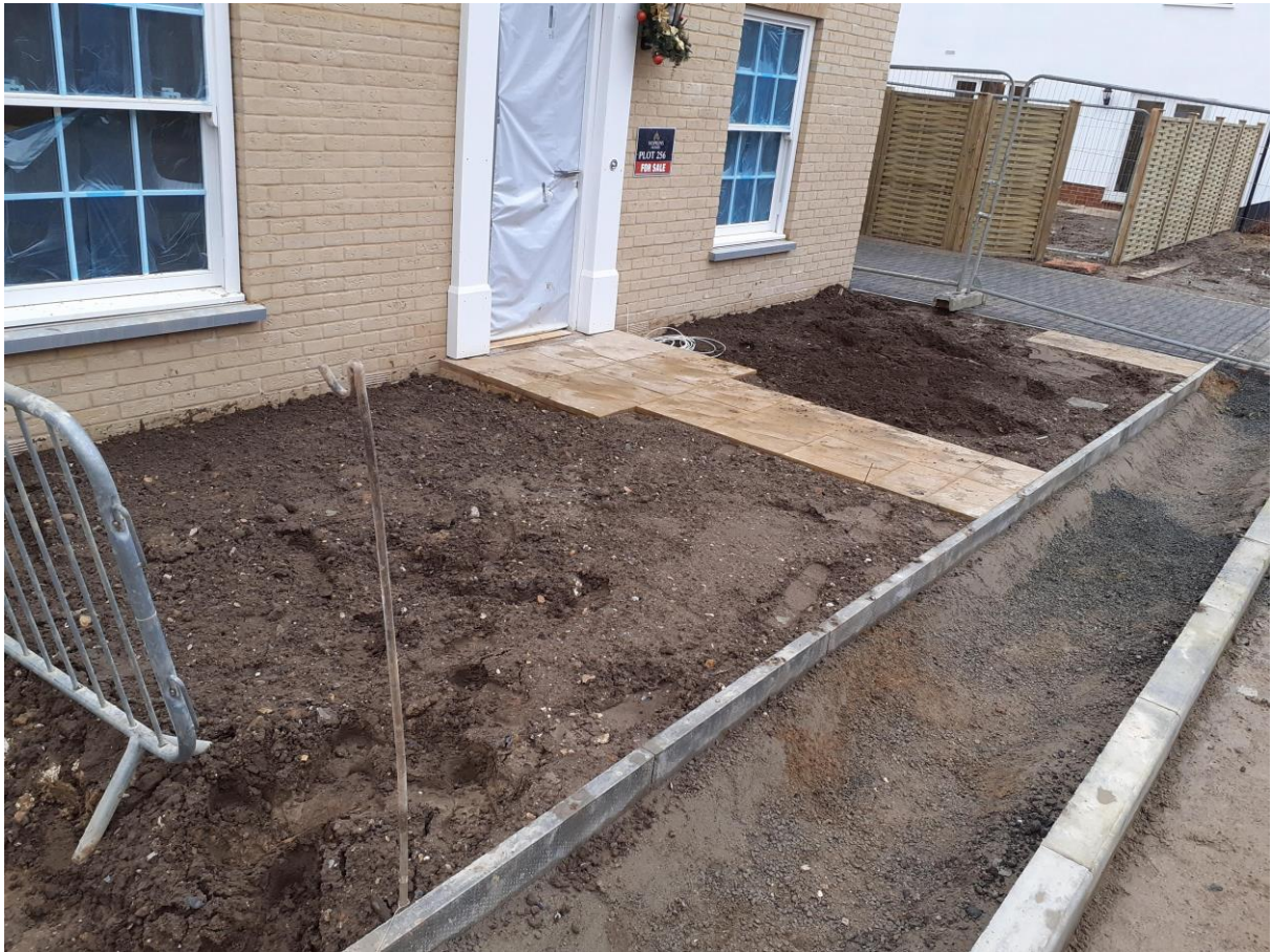
Photograph 5 , taken on the 19 th December 2019 by the client, showing completed cover system in the front garden of plot 256.
