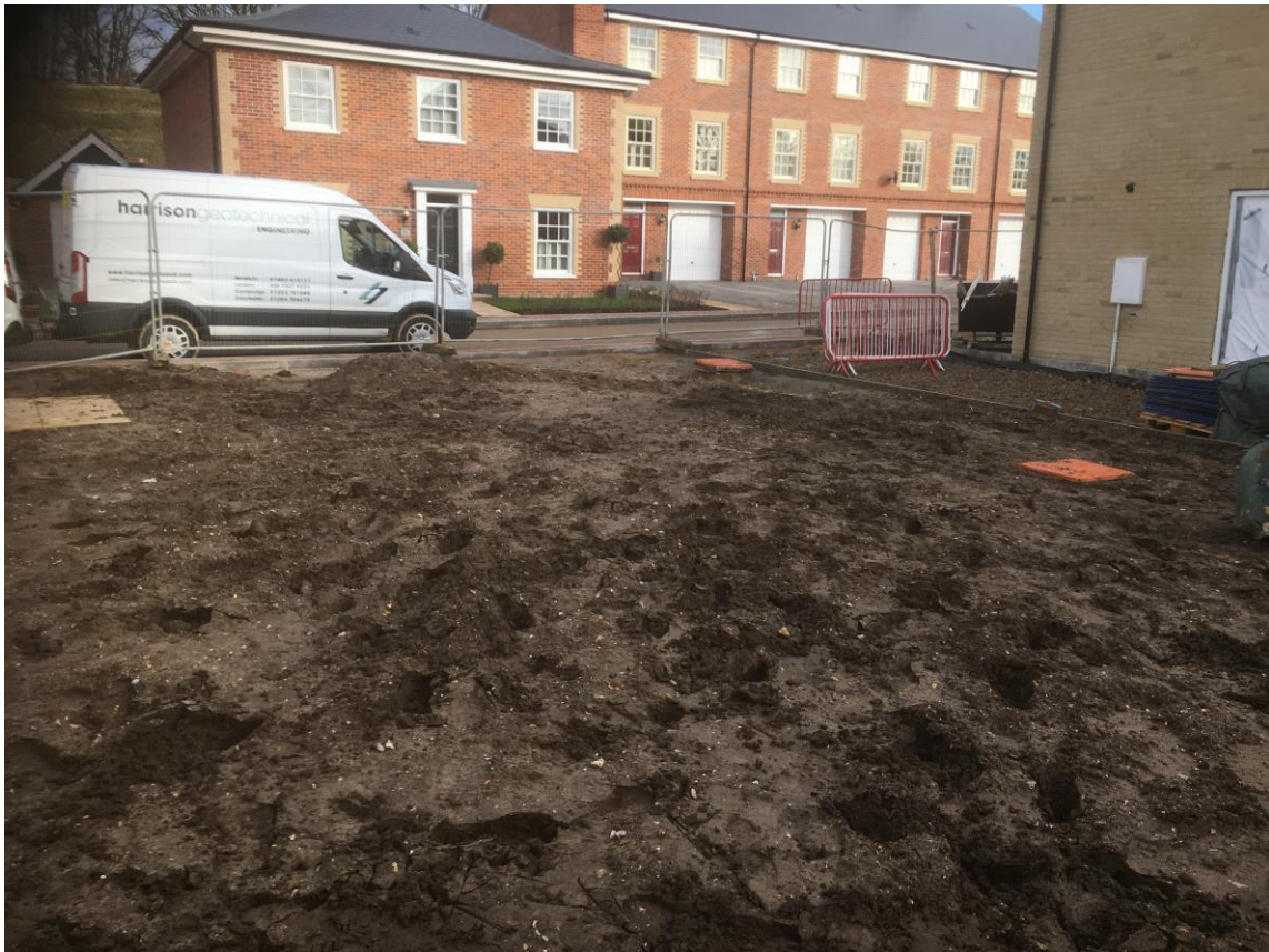
Photographs 1 - 3 , taken on the 3 rd December 2019, showing the depth and nature of subsoil and topsoil within the garden area of plot 259 (HDTP259-02) and the arisings generated.
