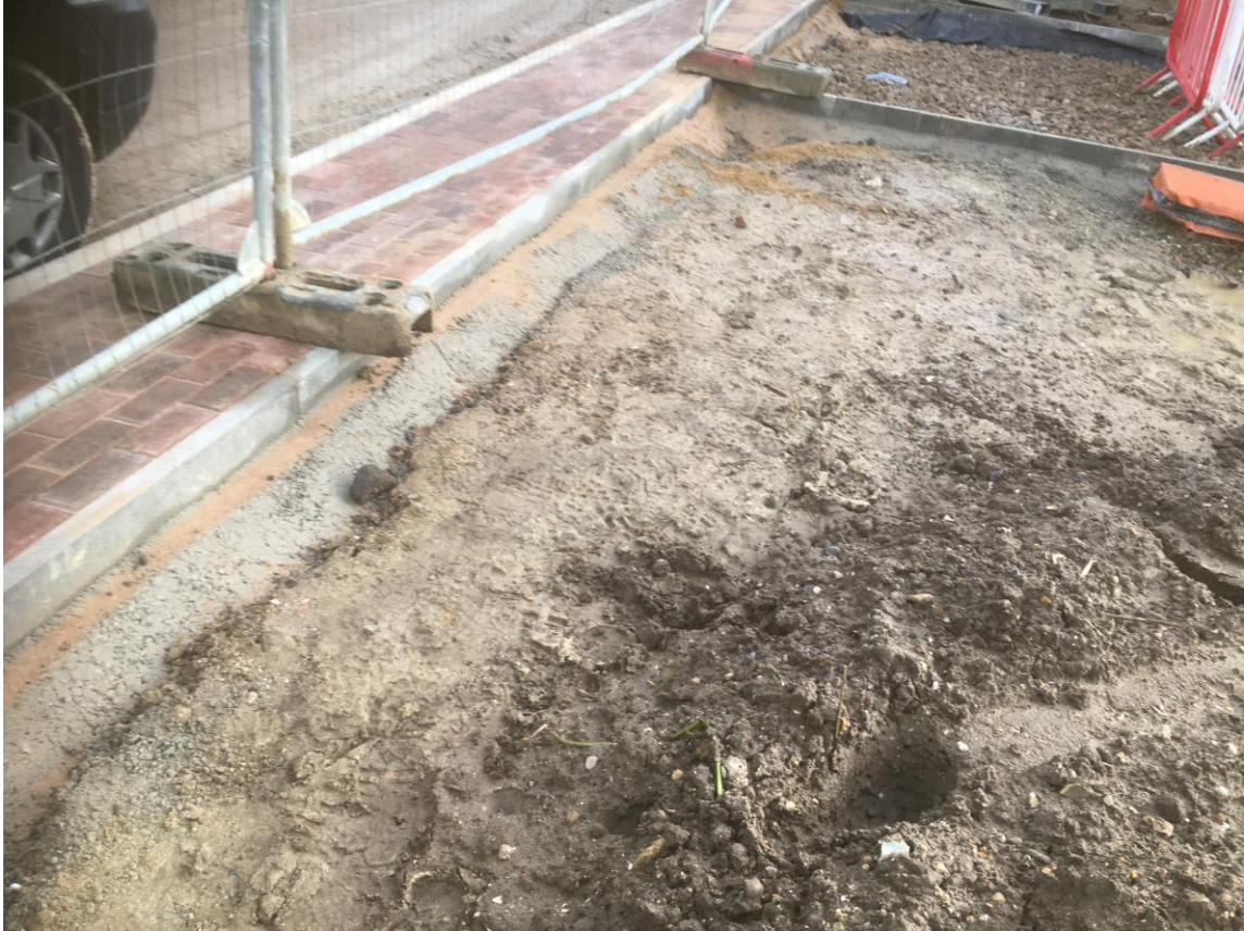
Photograph 4 , taken on the 3 rd December 2019, showing where the cover system was not present adjacent to footpaths and paving in plot 257.
