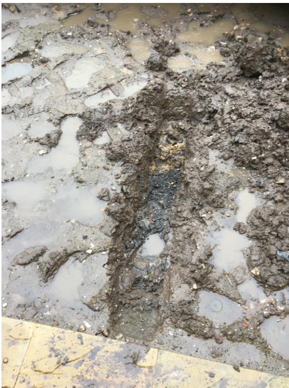
Photograph 7 , taken on the 5 th January 2021 showing the black material extending away from the paved footpath in plot 7.
