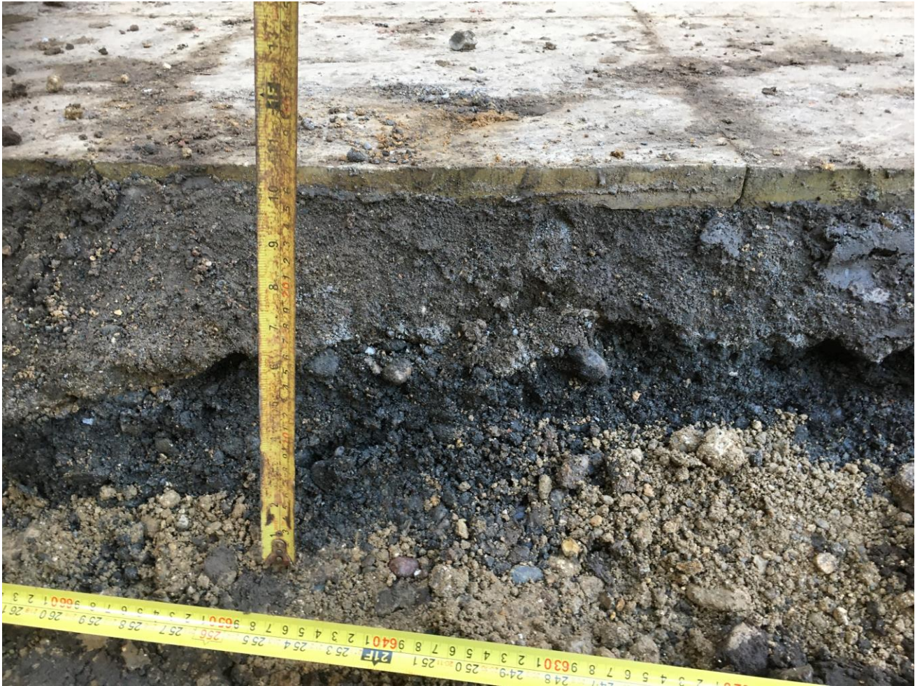
Photograph 9 , taken on the 7 th January 2021 showing the black material found as a subbase underlying the paved footpath in plot 7. A concrete apron was observed extending at approximately 45° from the footpath which generally capped the subbase material.
