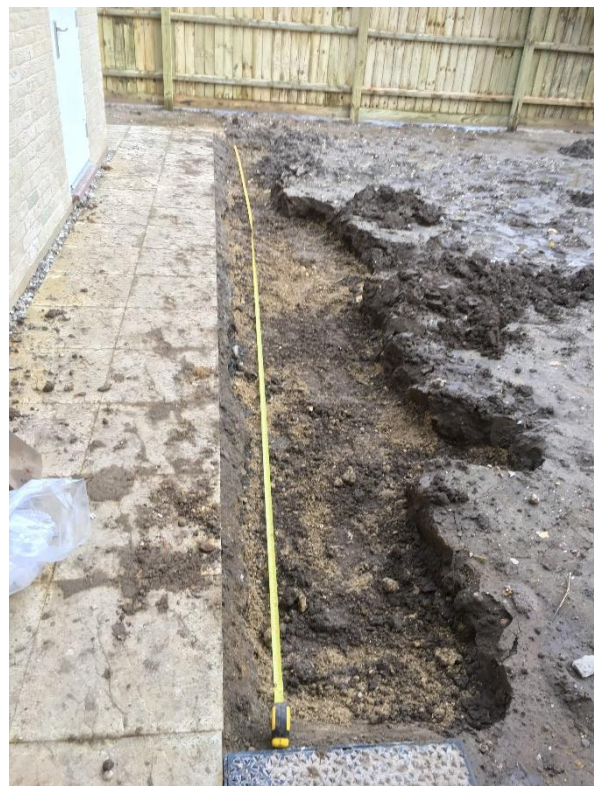
Photograph 8 , taken on the 7 th January 2021 showing the excavation of the black material encountered in plot 7.
