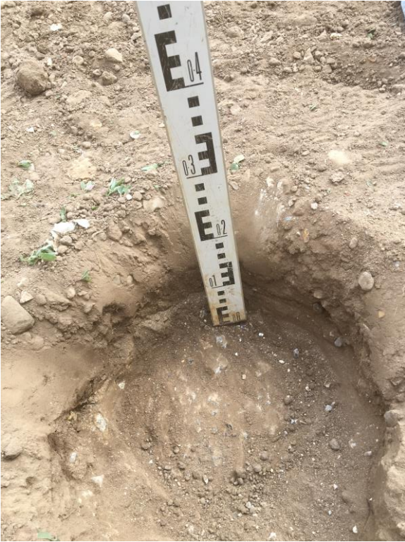
Photographs 5 , taken on the 2 nd September 2019, showing the depth of the concrete obstruction within the front garden of plot 169 (HDTP169-01).
