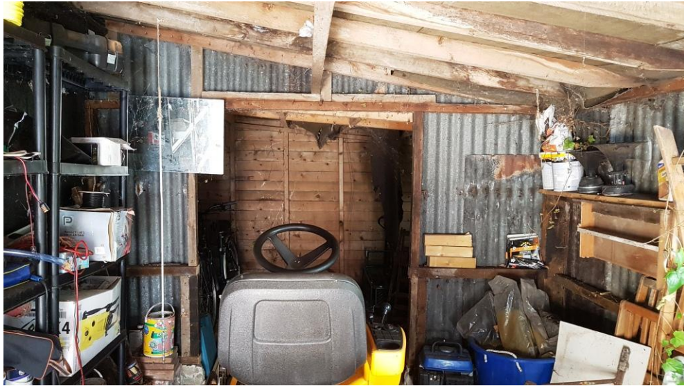
Existing lean-to is of very poor quality construction.
