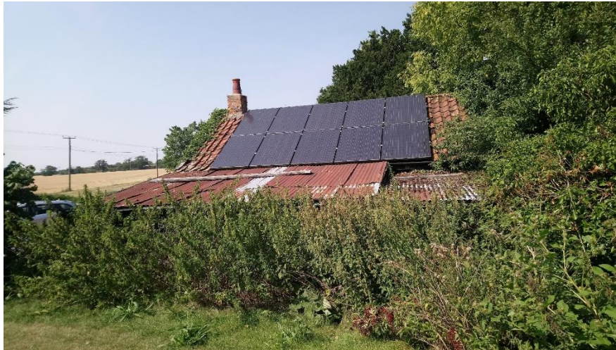
Corrugated roof of existing lean-to structure, old forge building beyond, from garden.
