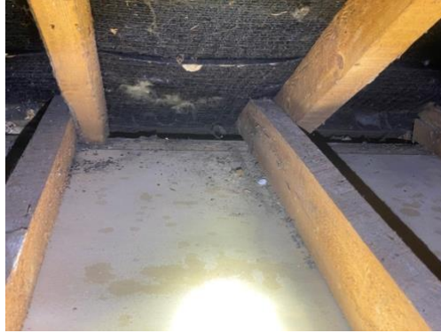
Photograph 2: Droppings in south-west corner
