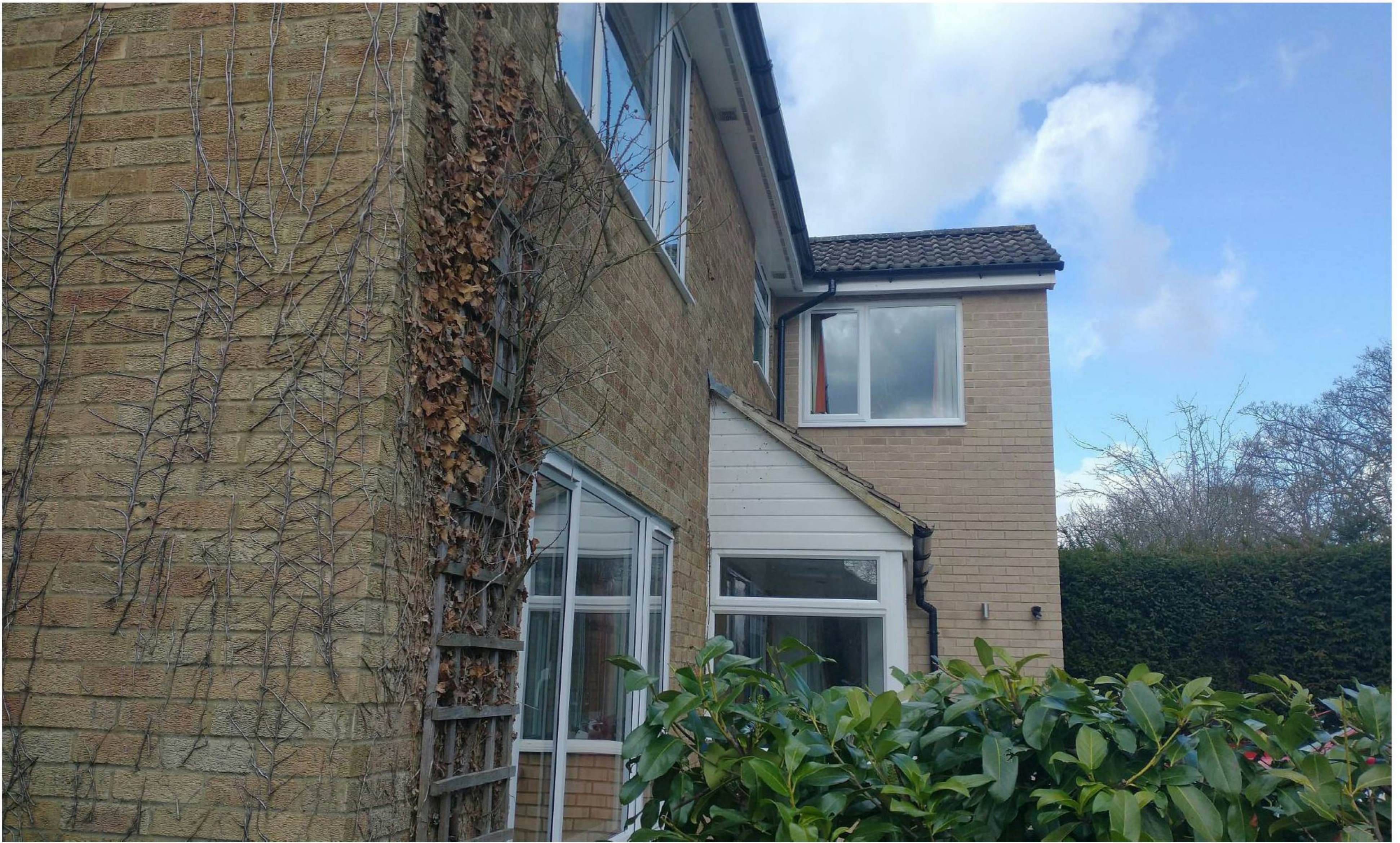
02 Flank elevation of No.44 Franklin Road – showing openable, first floor window facing South East with clear glass. Planning Permission 16/00131/FUL refers.
