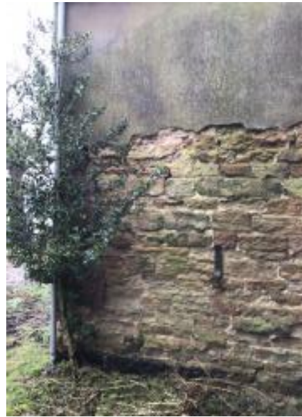
Stonework on the South West wall. Poor section to the top left behind the holly
