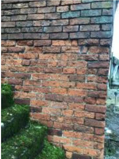
Badly eroded brickwork on the South East wall. This also shows them deeply eroded mortar
